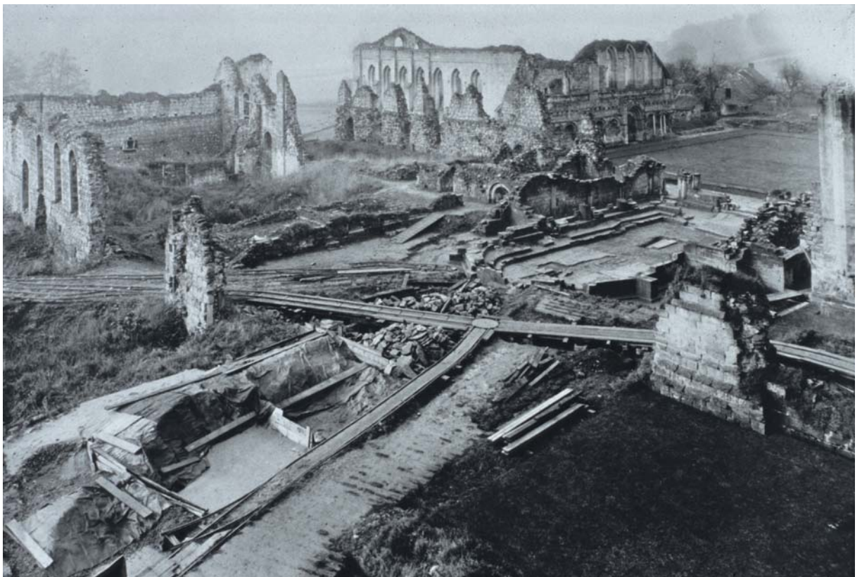
Site clearance in progress at Rievaulx Abbey in about 1921. Such was the scale of the works that a light railway system was used to transport spoil from the site.
