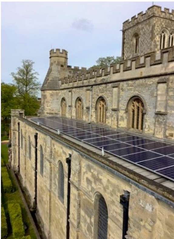
Figure 1. Photovoltaic panels on south aisle of Dunstable Priory © Diocese of St Albans and Dunstable PCC
