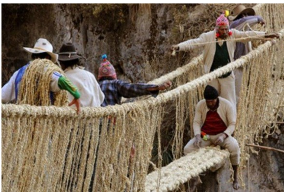
Image 2. Community restoration of the Inca bridge, Quehue. The bridge was constructed originally by the Empire 500 years ago. © Ambito, 2021
