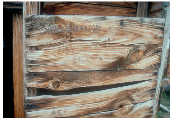
The effects of wind erosion on outer boards of Dedrick's hut cause deep grooves in the wood. The less dense earlywood cells of the wood are eroded faster than the latewood cells resulting in a grooved appearance. An inscription, "CHIEF SIGNAL OFFICER/WASHINGTON DC USA" placed on this reused wood during the Greely expedition (1881) has partially resisted the effects of the wind.
