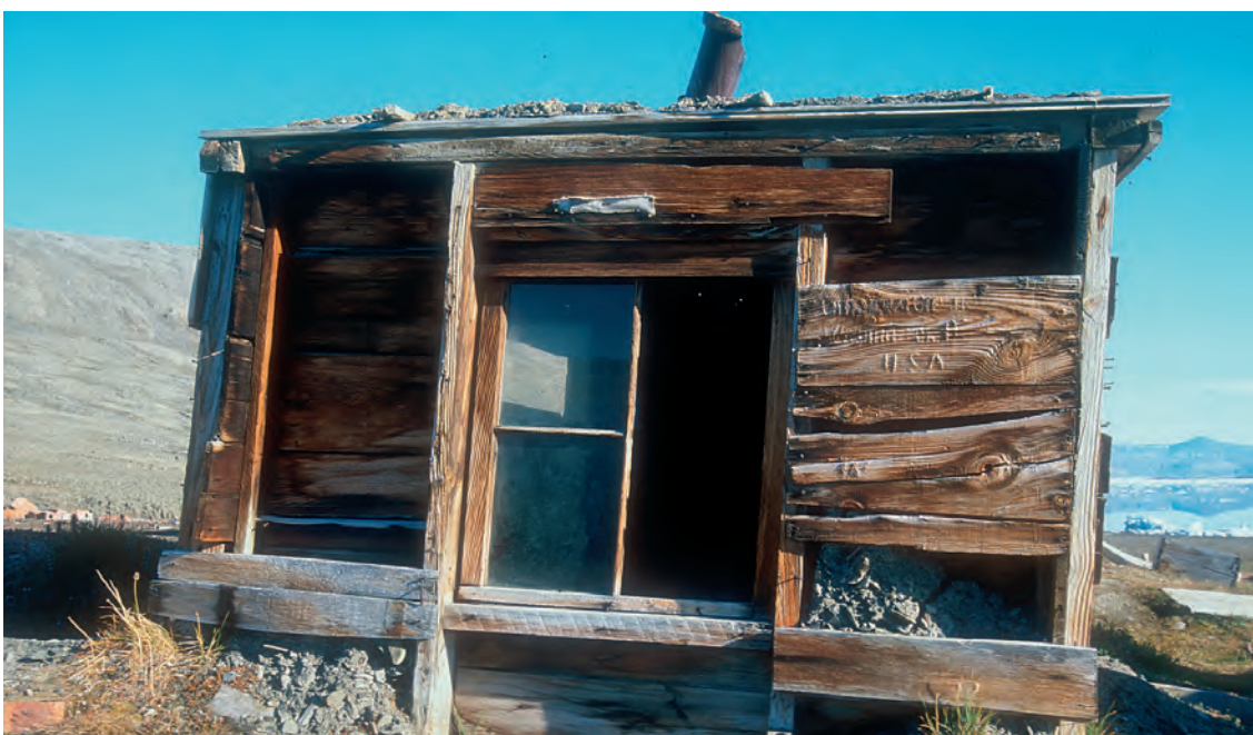
The Dedrick hut at Fort Conger. All three hut structures used by the Peary expedition have had serious deterioration over the past decades and the degradation processes continue unabated. Outer boards of the hut's multi-layered wall construction have blown off, windows and doors are open and the roof has blown off one hut. Non-biological deterioration (wind erosion and salt corrosion) as well as decay by wood destroying fungi has severely affected the wood in the huts.
