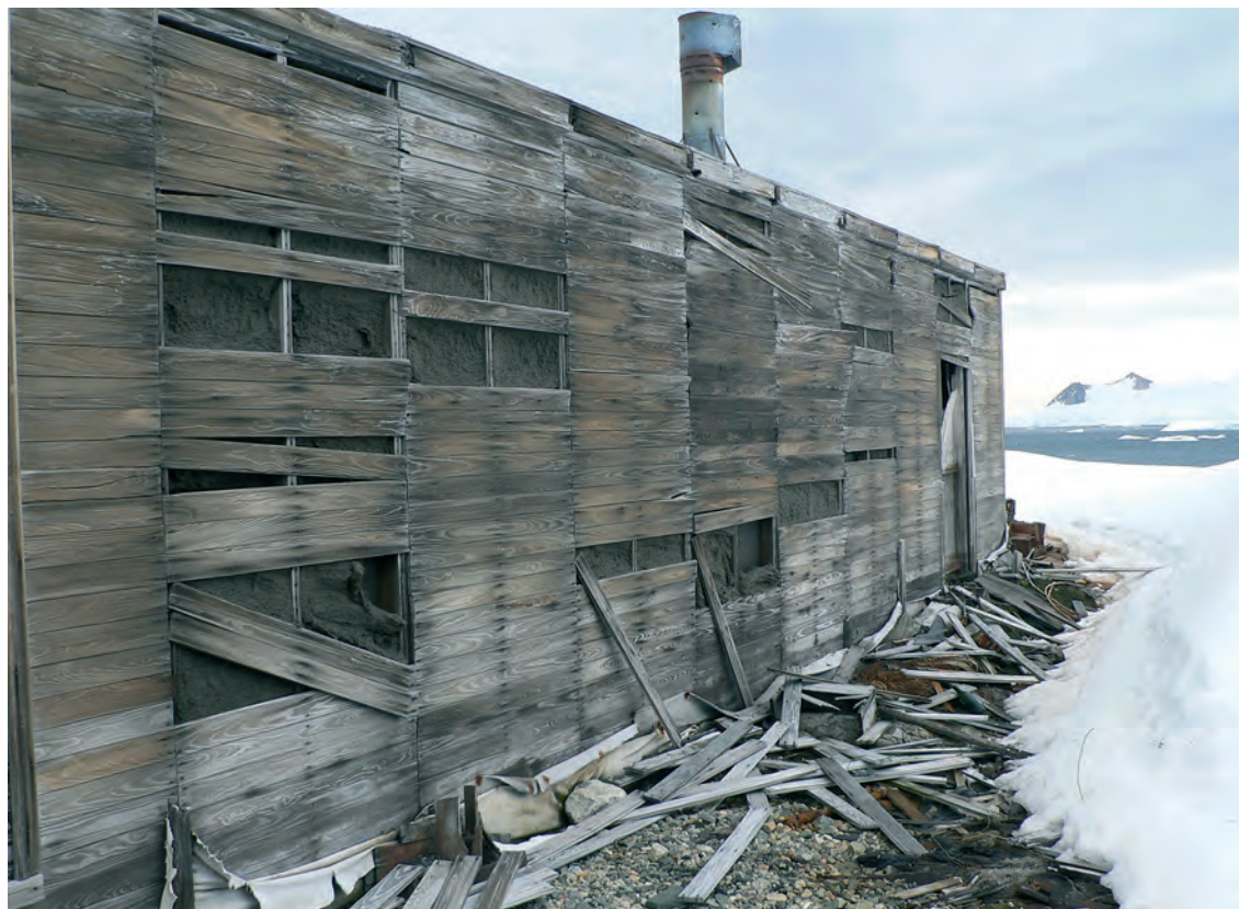
Fig. 3. Exterior north wall of the Main Building showing the loss of many wall boards. Photo: Brett Arenz
