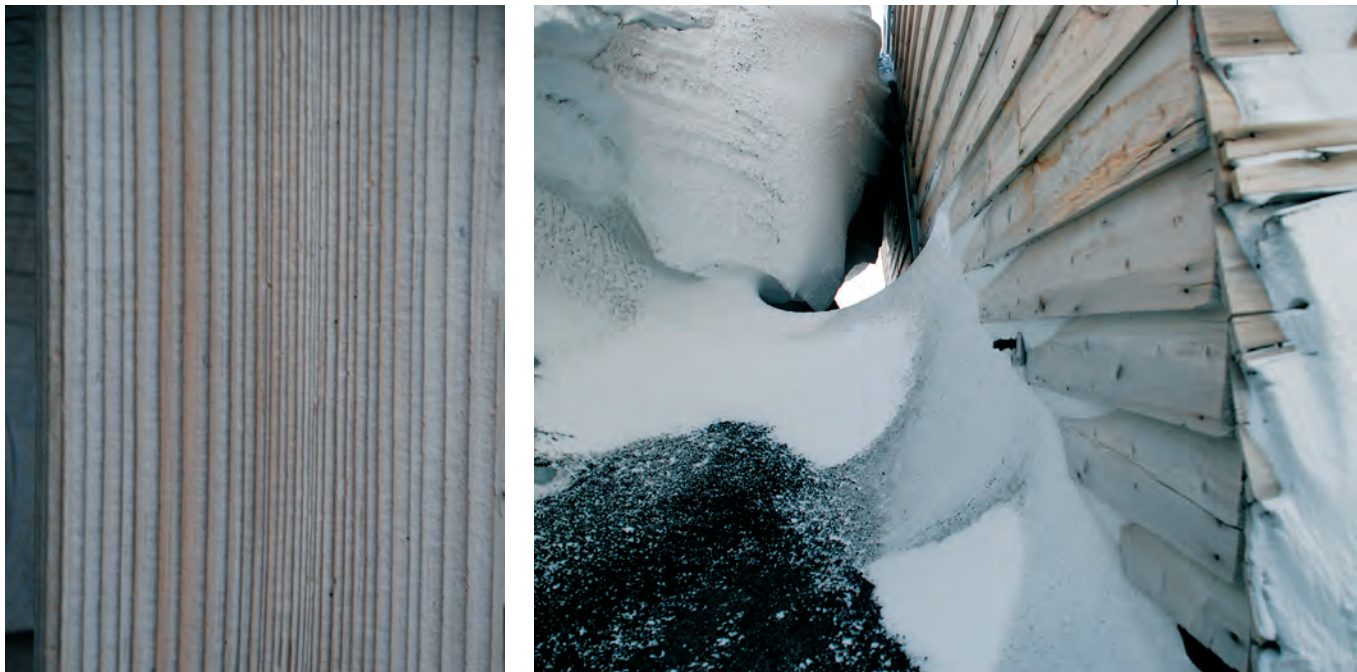
Evidence of affected wood at Terra Nova hut at Cape Evans: on the right it shows at the base of the exterior walls with the furrowed appearance of the wood surface due to salt erosion and on the left the evidence of selective removal of thin-walled earlywood cells. Photos: Roberta Farrell.
