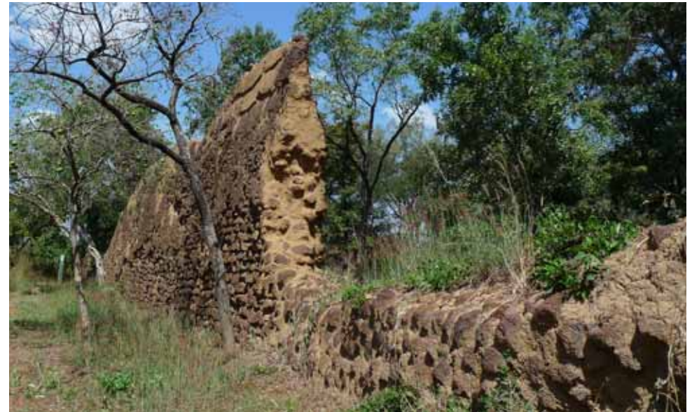
Tear on west wall © David Gandreau, CRAterre
