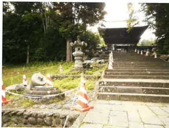
Figure 2.18 Collapse of stone lanterns at the Toshogu Shrine, Sendai City, an important cultural property
