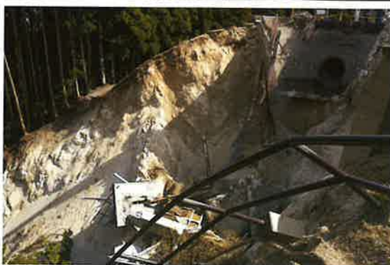
Figure 2.24 Ishioka Electric Power Plant (Top: Before earthquake; Bottom: After earthquake) (Ishioka city, Ibaraki Prefecture)
