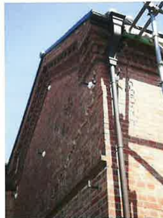
Figure 2.21 Disaster-affected brick storehouse, the Machikado Kura Nomura (Top: Building exterior; Bottom: Cracked gable wall)
