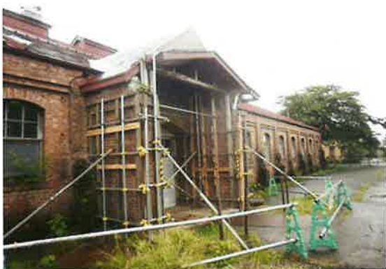
Figure 2.20 Disaster-affected modern heritage, the former covered parade ground building
