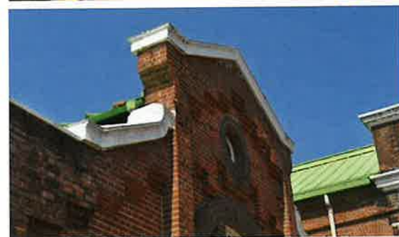
Figure 2.22 Disaster-affected Chateau Kamiya winery building, an important cultural property Top: Building exterior; Bottom: Cracked gable wall)
