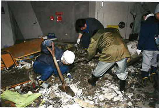
Figure 3.4 Salvage activities at the Ishinomaki Cultural Center
