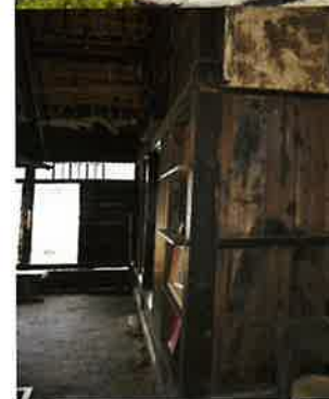
Figure 2.8 The important cultural property, the former Baba Family Residence, which is tilting (Top: Exterior; Bottom: Tilting interior)
