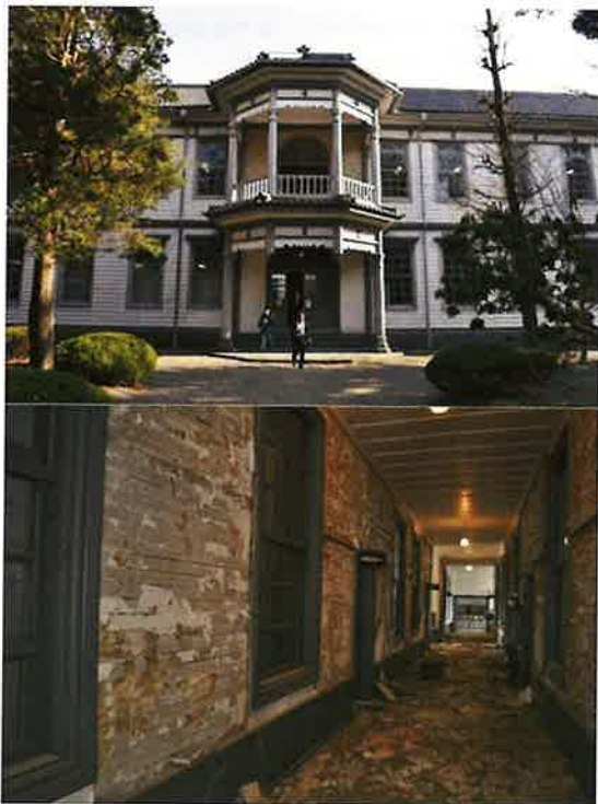
Figure 2.9 Damage to the important cultural property, Fukushima Prefecture Jinjo Junior High School (Top: Building exterior; Bottom: Peeling lath wall)
