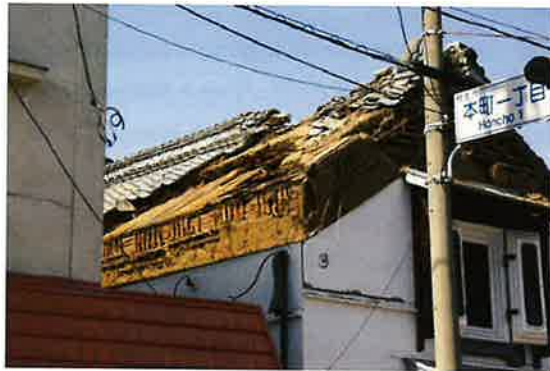
Figure 2.10 Damage to classic dozo (mud-wall warehouse) - the registered tangible cultural property, the Mori Goshi Gaisha storehouse
