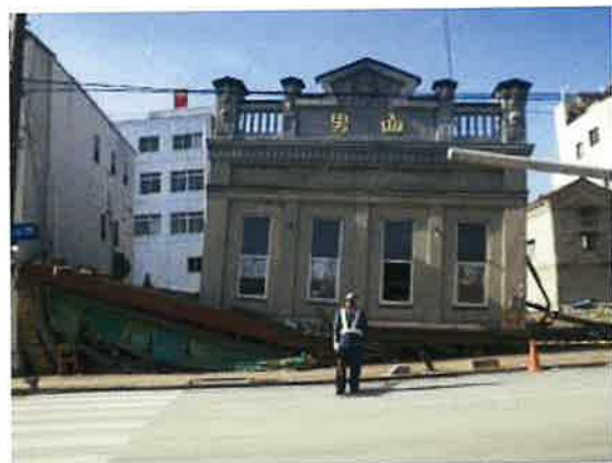
Figure 2.13 Tsunami-caused damage to the registered tangible cultural property, the Otokoyama Shuzo original store
