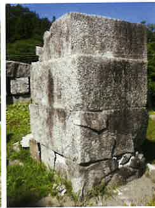
Figure 2.16 Displaced and cracked stone masonry at the Hashino Blast Furnace, a historic site in a Kamaishi City
