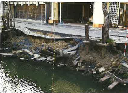
Figure 2.28 Historic riverside damaged
