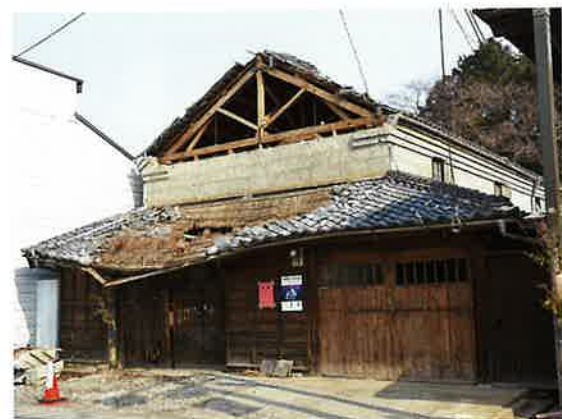
Figure 2.26 A damaged house in Makabe
