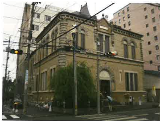
Figure 2.19 Former 99 Bank Head Office, an important cultural property: Minor damage to internal walls and ceiling
