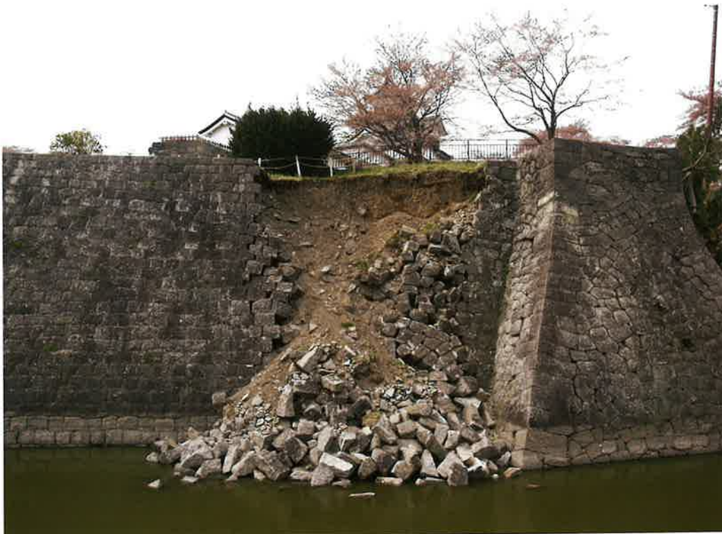
Figure 2.30 Collapsed masonry walls of Komine Castle
