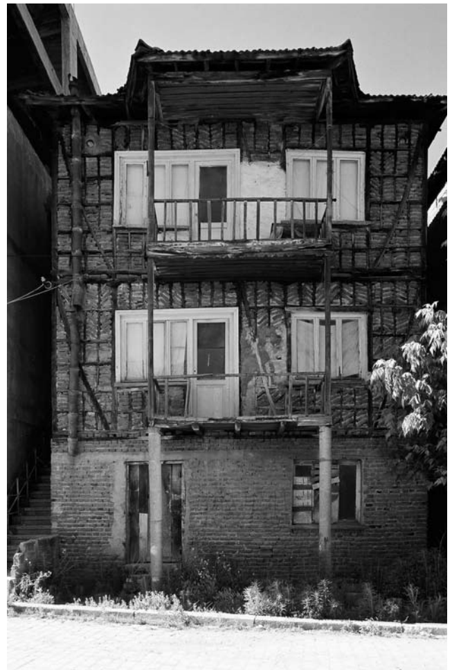
Fig. 5 This three story house in Gölcük located less than one km from the fault was undamaged by the 1999 earthquake, while a number of reinforced concrete buildings on the adjacent blocks collapsed (photograph © Randolph Langenbach)
