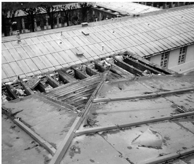
Fig. 1 Esquirol Hospital, building C, detail of the storm-damaged roof
