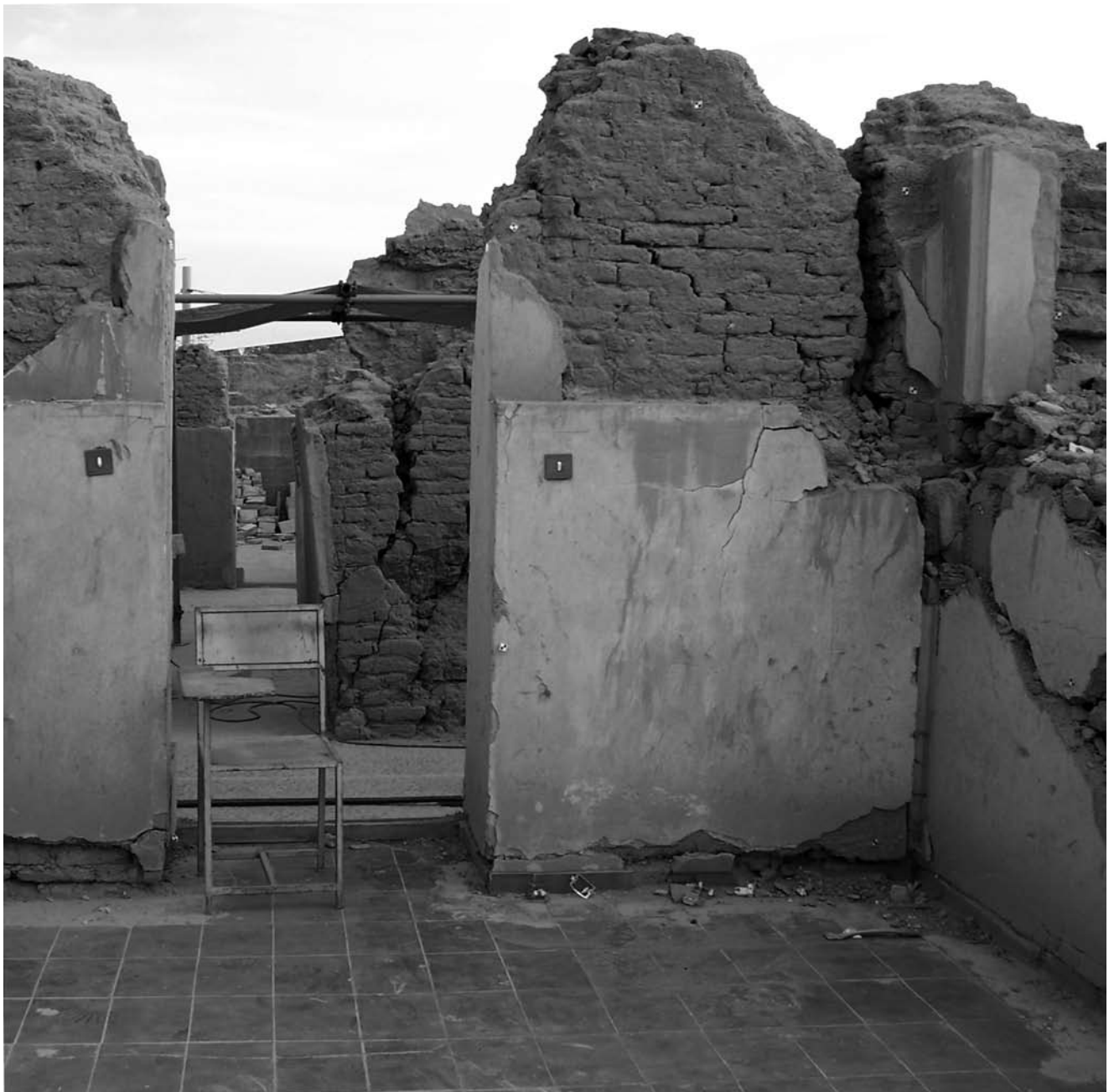
Bam Citadel, typical damages on masonry structures, loss of integrity (Wolfram Jäger)
