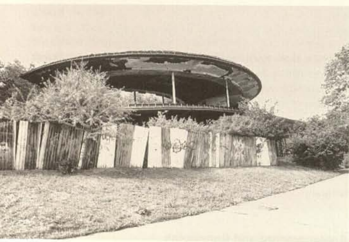
The EXPO 58 Restaurant: the exterior after devastation lasting several years - photograph from 2000
