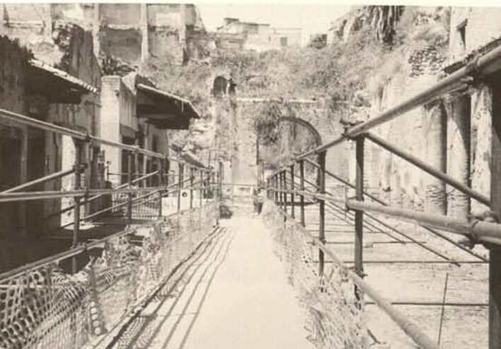
Both sides of the building fronts of the Decumano Massimo blocked off
