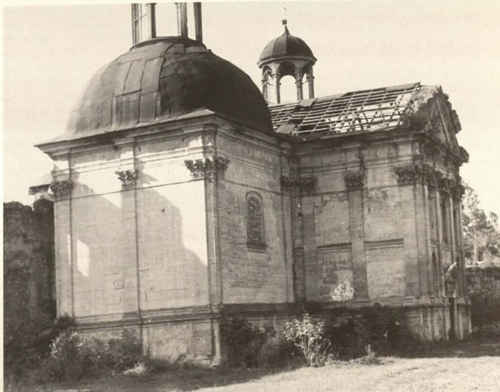
Palace of the Senyavski family in Berezhany, chapel of the late 17 th century in decay
