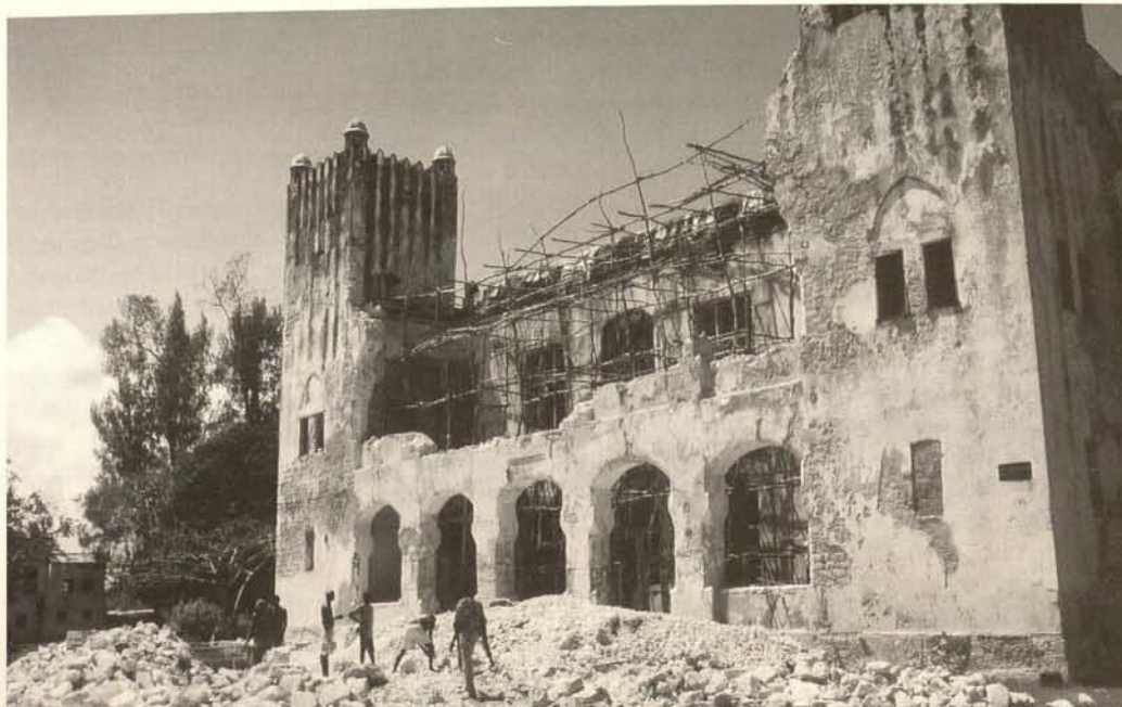
The Boma after December 2000: dangerous parts of the façade had to be taken down. Will it be possible to reconstruct it soon?
