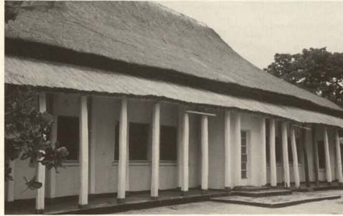
Barotse Royal establishment, Litunga's winter palace, Lealui, built in 1902. The roof has been severely attacked by termites.
