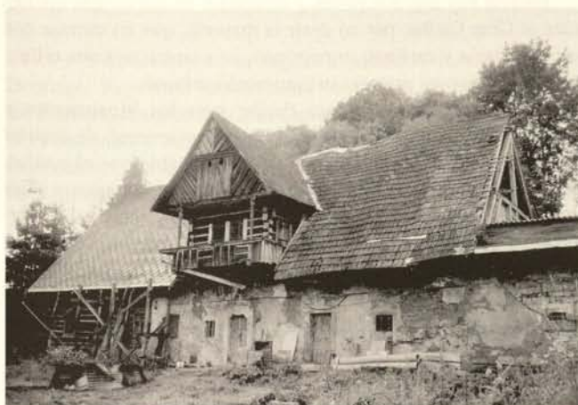
Havlovice, land-register No. 36, District of Trutnov - a timbered farm from the end of the 18th century in a critical state
