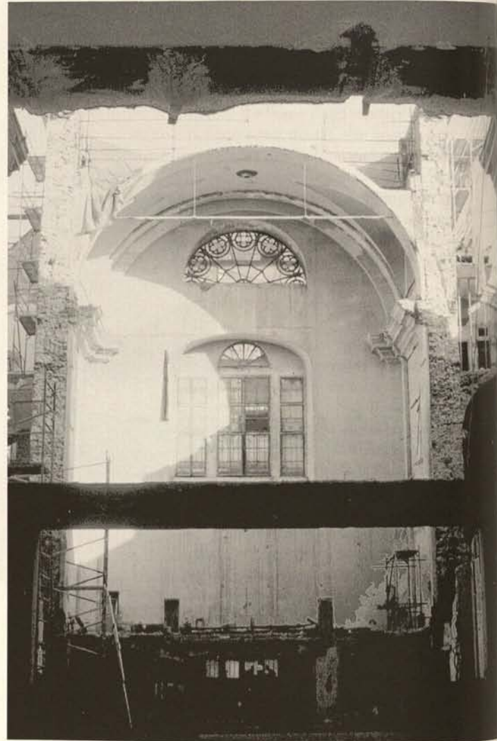
Praha 1 - the New Town, the U Hybernů House: the interior of the nave of the former church after its partial demolition, photograph from 2000
