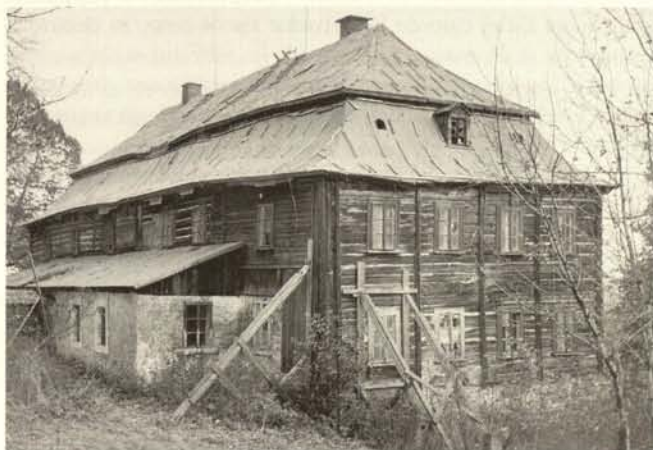
Krásná, land-register No. 10, District of Jablonec nad Nisou - a massive timbered house built in the mid-18th century, its present state being critical
