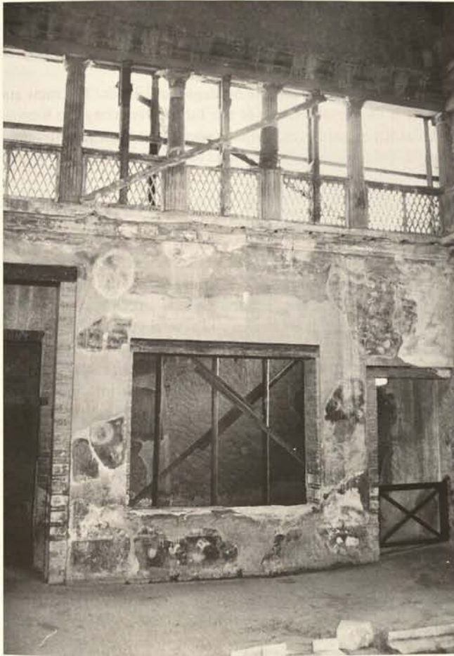
Casa sannitica: provisionally supported ceilings and severe water damages due to leaking roof
