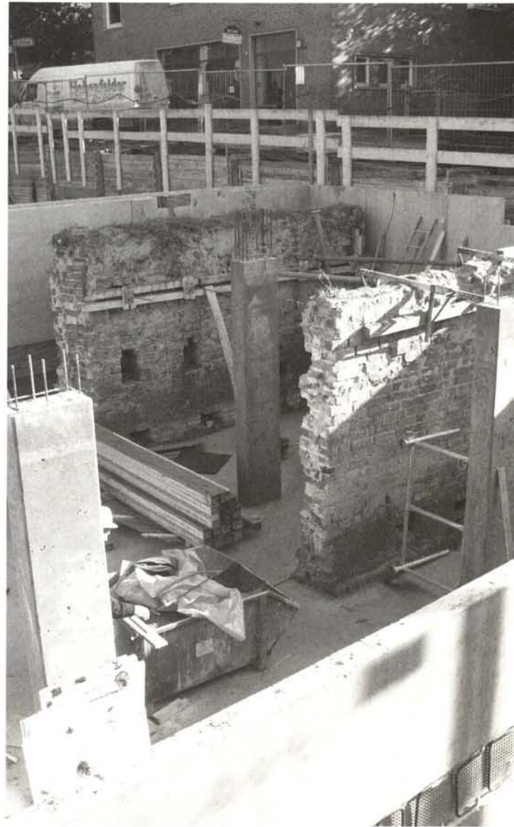
Preserved Gothic walls in the basement of the planned hall of residence (photo: Fröhlich/Reck)
