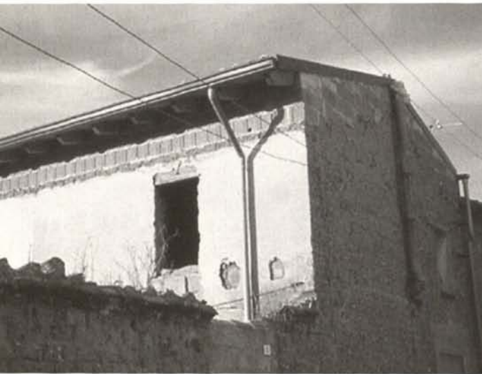
The top part of this earthen building shows repair with cement blocks (Terralba, Sardinia)
