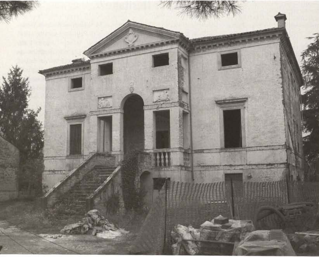
Villa Forni-Cerato in Montebelluna near Treviso, a building by Andrea Palladio (1541-2). A piece of World Heritage in an increasing state of decay (leaking roof, no windows, the dilapidated interior with endangered wall paintings).
