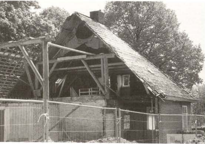
A farm in reconstruction, showing the traditional structure. Will the result of this building activity meet the standards of the Venice Charter?
