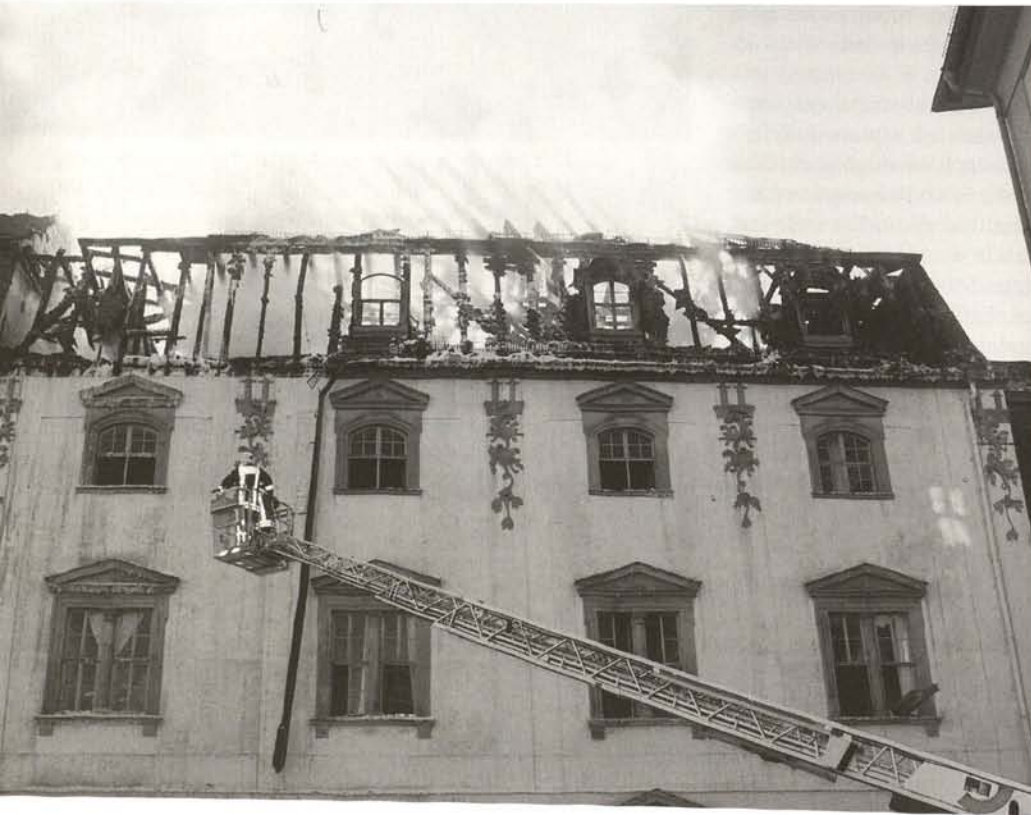
Weimar, Anna Amalia Library, west facade on the day after the fire (3 September 2004), smouldering fires not yet extinguished (photo: J. Seifert)
