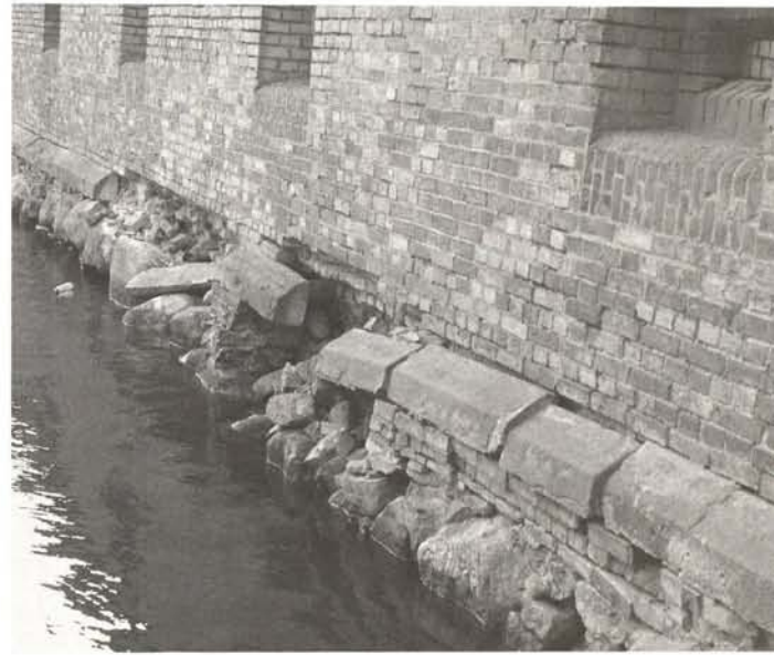
Vistulamouth Fortress in Gdansk, the brick bastions in need of conservation work
