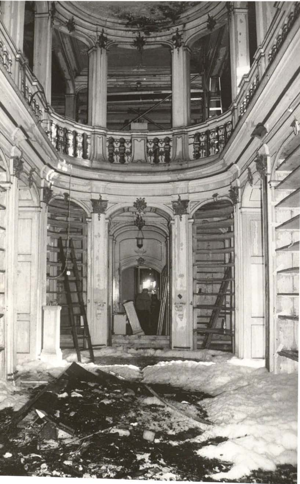
The cleared-out Rococo hall after the fire with remains of debris and foam as well as with provisional shoring (photo: J. Seifert)
