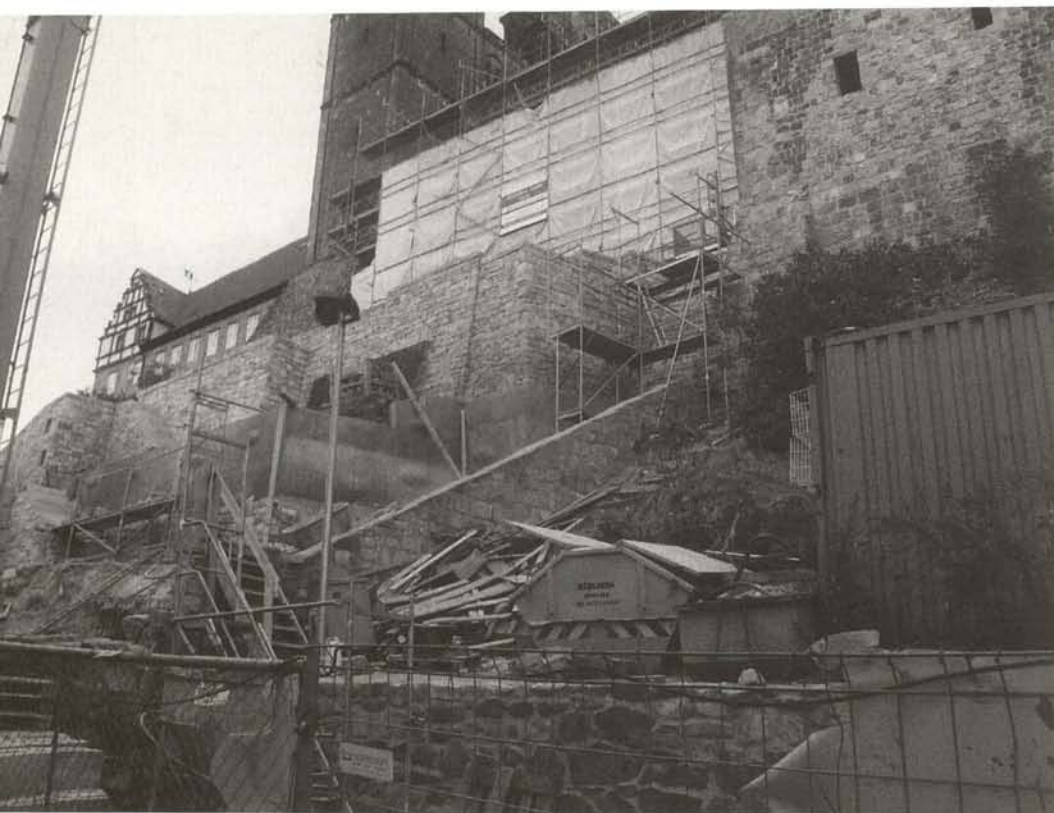
Quedlinburg, so-called Schlossberg, southern wall underneath the convent church during repairmeasures, October 2004 (photo: A. Hubel)
