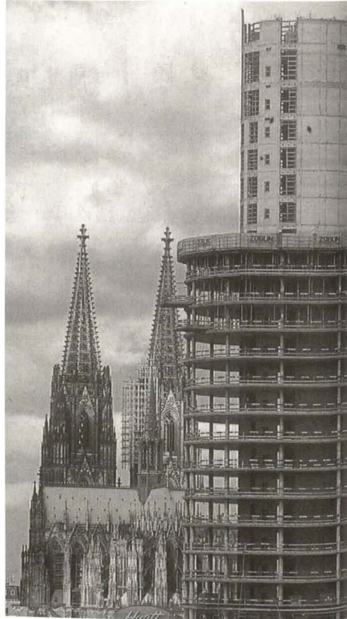
Cologne, the RZVK building during construction with the cathedral in the background
