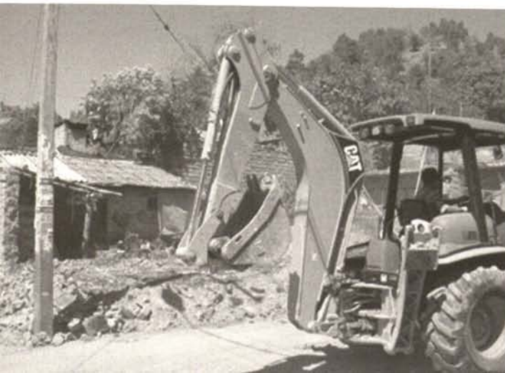
Destruction of adobe buildings in Hueyapan (Morelos)
