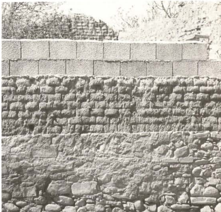
Misrepair of an earthen wall by means of cement blocks (Ussana, Sardinia)
