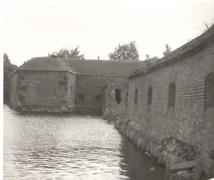
Vistulamouth Fortress in Gdansk, view on to the damages of the bastion's bricks caused by water
