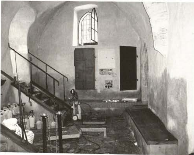
The southern hallway is the oldest addition to the Synagogue, it originated, evidently, already during the construction in the last quarter of the 13 th century. The condition shortly after the falling off of water during the 2002 flood.
