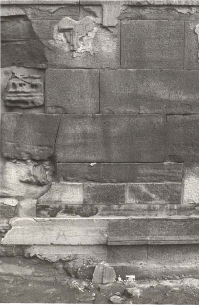
Qasr al Bint, condition of stucco decoration
