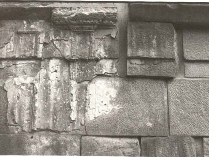
Qasr al Bint, recent rupture on stucco decoration
