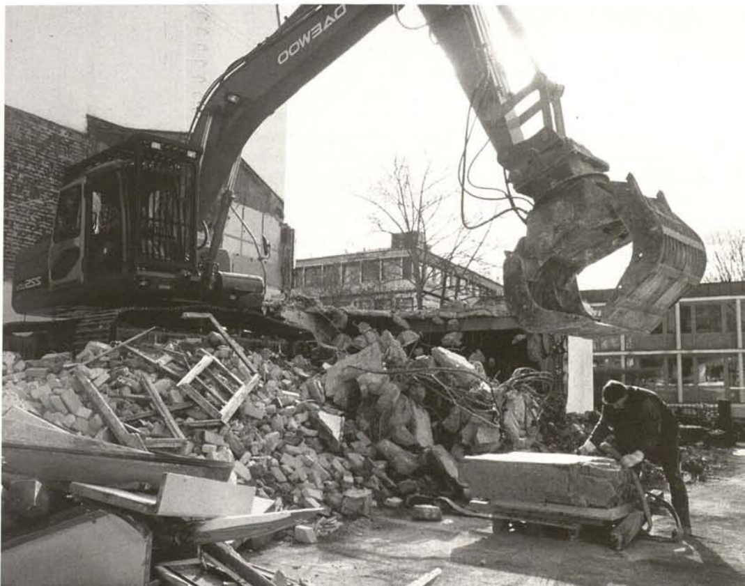
The demolition contractor rescues a remaining piece of wall with traces of the Gesamtkunstwerk
