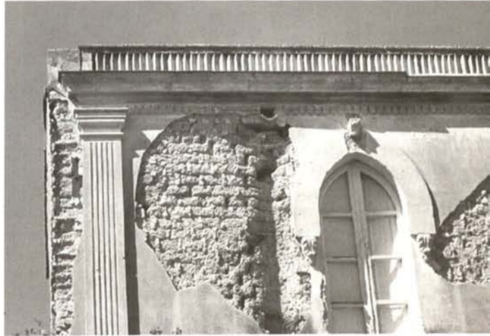
Erosion of mudbrick caused by neglect and lack of maintenance of downpipes and gutters (Samatzai, Sardinia)
