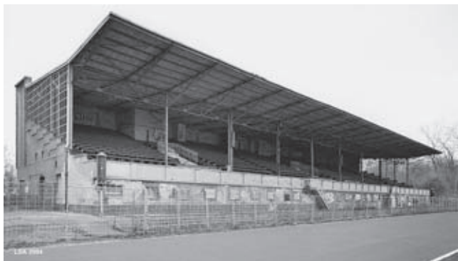
Poststadion, Berlin, 1926–29, arch. Georg Demmler, listed monument. Out of use since the beginning of the 1990s. Condition c. 2000
