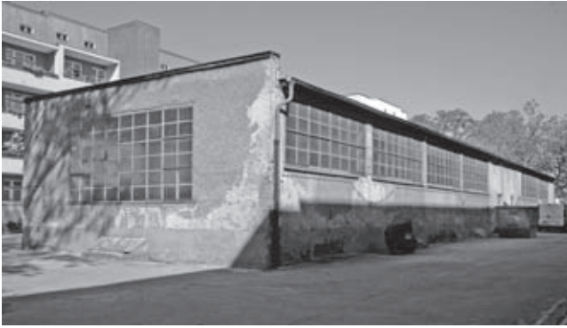
Wohnstadt Carl Legien, Berlin, 1928–30, arch. B. Taut, F. Hillinger, listed monument. Out of use since the beginning of the 1990s. Current condition of the laundry house which is threatened by an application for demolition
