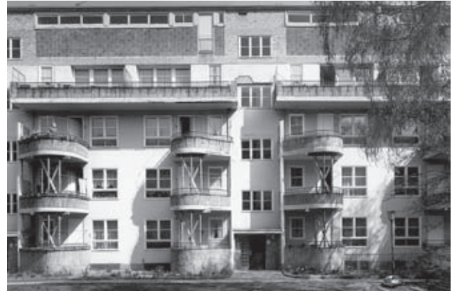
Siemensstadt. Row houses by Hugo Häring. Balconies before restoration
