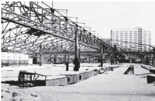
Bakhmet'jevsky-Park bus garage, Obraszova Street 19a, Moscow; arch. K. S. Melnikov, 1926–27, monument of local importance. The roof trusses were illegally removed in 2002
