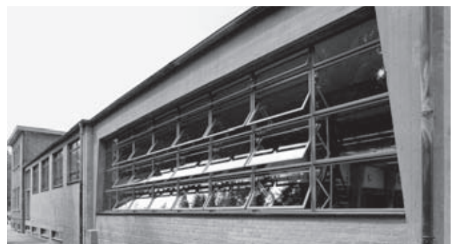
Former school of the German Trade Union (ADGB) in Bernau near Berlin, window of the refectory after reconstruction 2006
