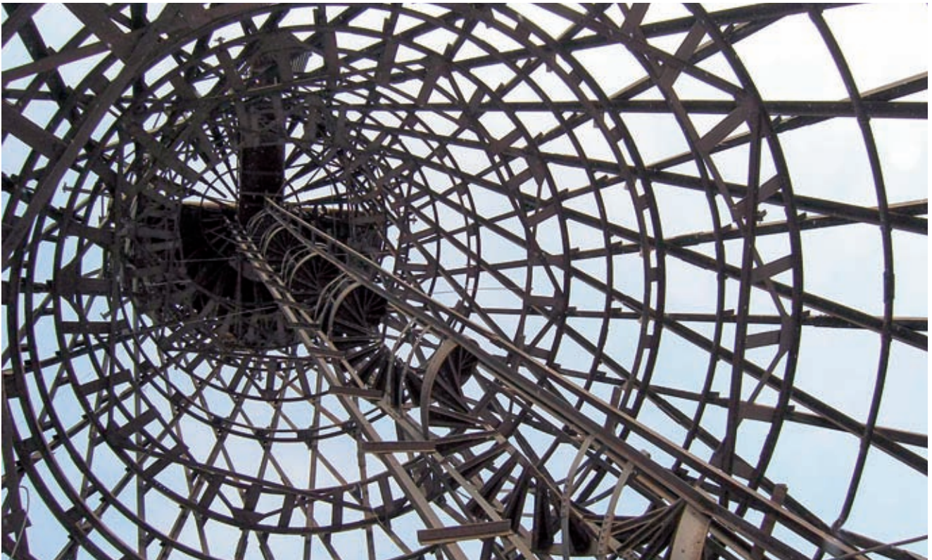
Watertower in Vyks in the Nizhnij Novgorod region. Present condition. Credit: S. Zelenova, Nizhny Novgorod
