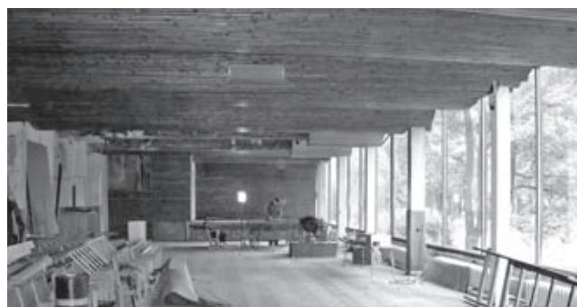
Viipuri Library, arch. A. Aalto, 1927–35. View of the Lecture Hall during the restoration works in 2003
