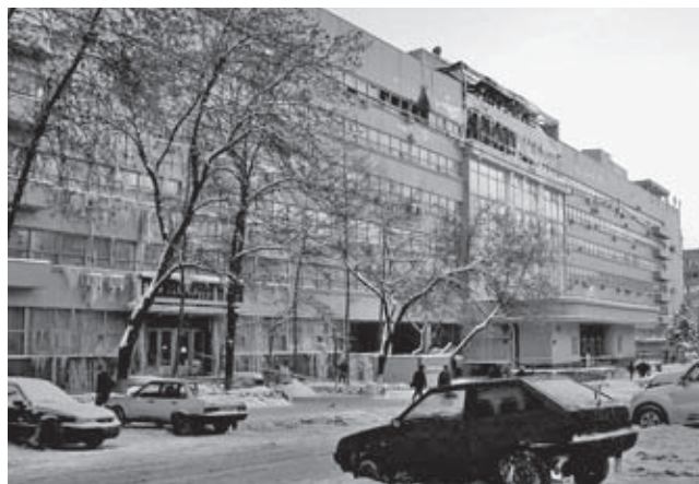
Pravda – printshop and publishing house, Pravda street 25/4, Moscow, arch. P. A. Golosov and A. V. Kurovsky, 1930–35, monument of local importance. View from Pravda street after the fire in february 2006
