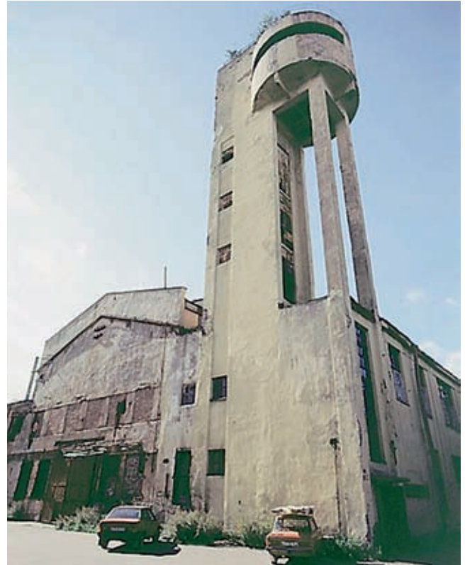
↑ Watertower of the "Krasny Gvozdilshchik" Cable Factory in St. Petersburg, 1930–1931, arch. J. Chernikhov. Condition in 2005. Credit: M. Stiglitz. Photo: V. Egorovsky, V. Lelina, A. Pastukh
