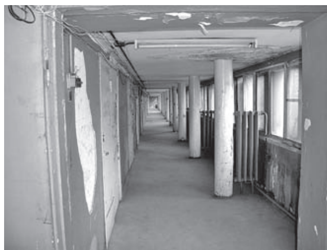
Narkomfin Commune House, Moscow, 1928–30, arch. M. Ginzburg, I. Milinis. One of two corridors giving access to the five upper floors of the apartment block, 2004
