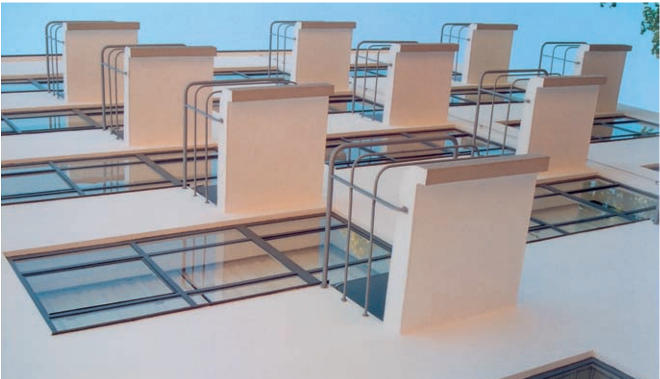
Bauhaus Building in Dessau, arch. W. Gropius, 1925. Balconies of the dormitory after the restoration. Current condition. Credit: Bauhaus Dessau Foundation. Photo: K. Baumann
