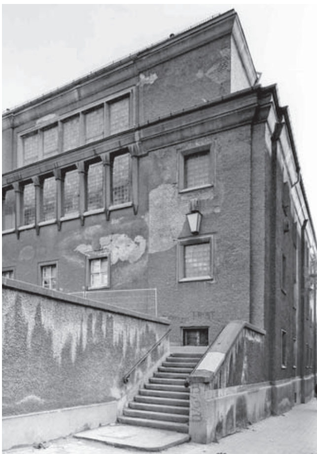
Hubertusbad, Berlin, 1925–27, arch. Rudolf Gleye, Otto Weis, listed monument. Out of use since the beginning of the 1990s. Condition c. 2000
