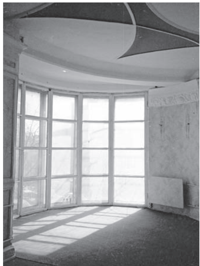
Burevestnik workers club, Moscow, 1927–29, arch. K. Melnikov. Clubroom before the restoration in 2000
