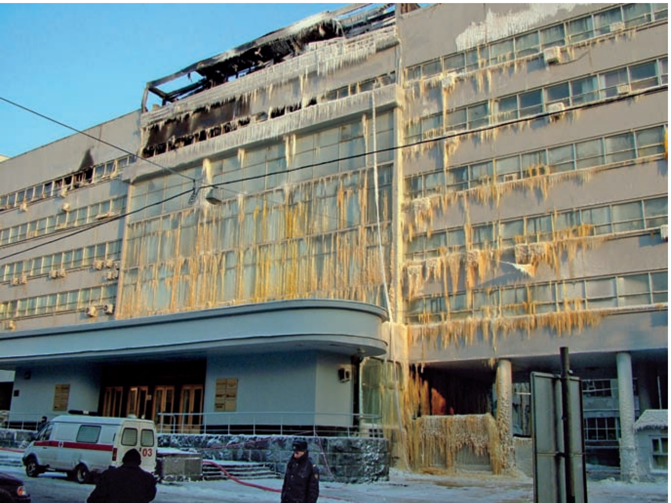
Pravda printshop and publishing house, Moscow, 1931–37, arch. P. A. Golosov, A. V. Kurovsky, monument of local importance. After the fire in February 2006. Credit: Schusev Museum of Architecture, Moscow. Photo: J. I. Rogozin
