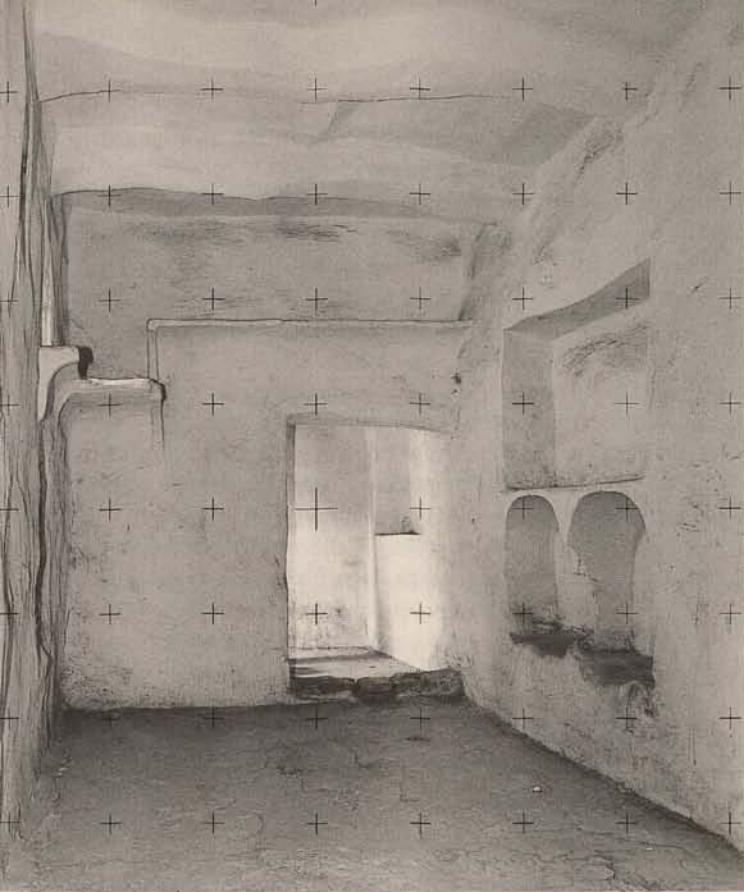
Abb. 12. Samsarat al Mansurah; 1. Obergeschoß, Musterraum; 1988 Fig. 12. Samsarat al-Mansurah; 2 nd floor, sample room; 1988
