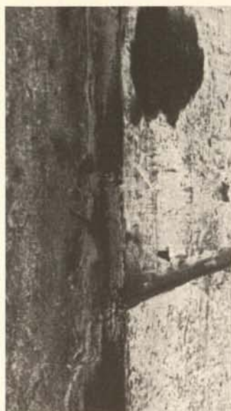
Fig. 2a, b. Copper roof of Queen Ann's Summer Palace (Belveder), built in 1558-1564; sheet with corrosion-mechanical defects
