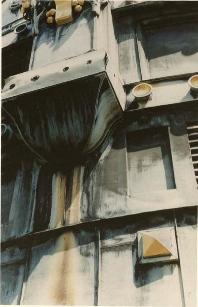
1. Prague, cupola of the Town Hall (Obecni dum), built in 1906-1911; corrosion of rivets of joints, deformation of the decoration box, leakage of water with rust
