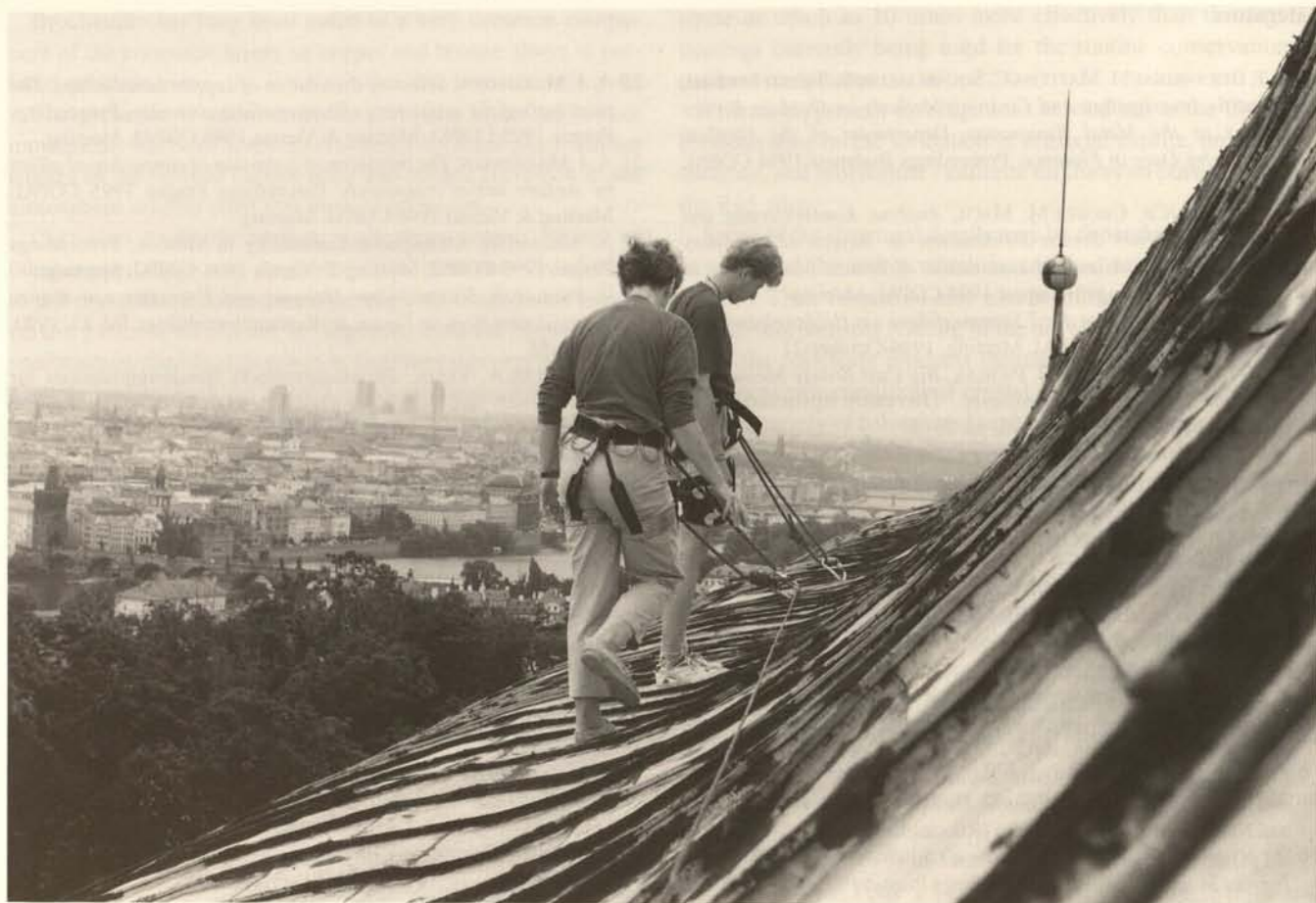
Fig. 1. Copper roof of Queen Ann's Summer Palace (Belvedere), built in 1558-1564; eastern ridge damaged part
