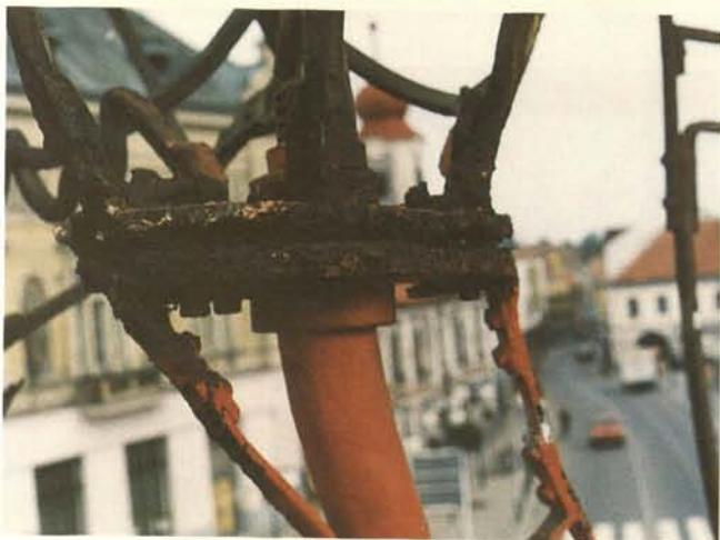
3a, b. Prague, equestrian statue of Jiri z Podebrad (J. Schnirch, 1890); corrosion damage of inner iron skeleton
