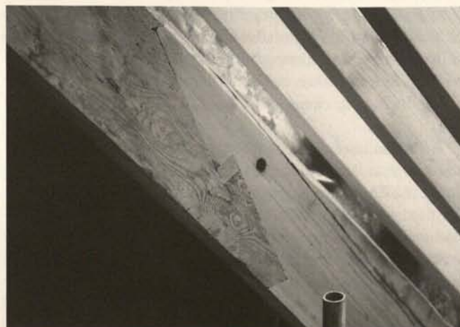
Fig. 9. Repaired Rafter. – By ‘scarfing’ a new piece of timber on to the bottom of this rafter it has been possible to retain most of the original 18 th century material. This type of repair is traditional in Britain, and very strong.
