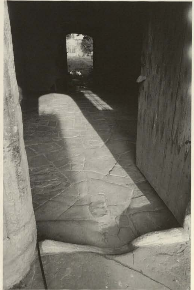
Fig. 12. Fourth case study: Acton Court. Cross passage floor from west to east after lime mortar repairs. Note the unusual configuration of pennant stone parving.
