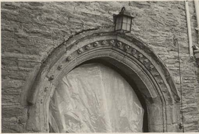
Fig. 8. Third case study: Broadfield Court. The fourteenth century doorway before repairs. Note decayed surfaces to hoodmould and surrounding rubblework, and Portland cement fillings.
