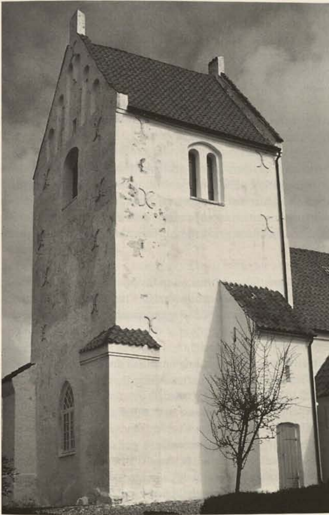
Fig. 7. Vallekilde Church (Zealand) 1996. The rendering has fallen off in the areas with cement and hard-burnt bricks. Repairs have later been executed with hydraulic mortar, which seems to hold.
