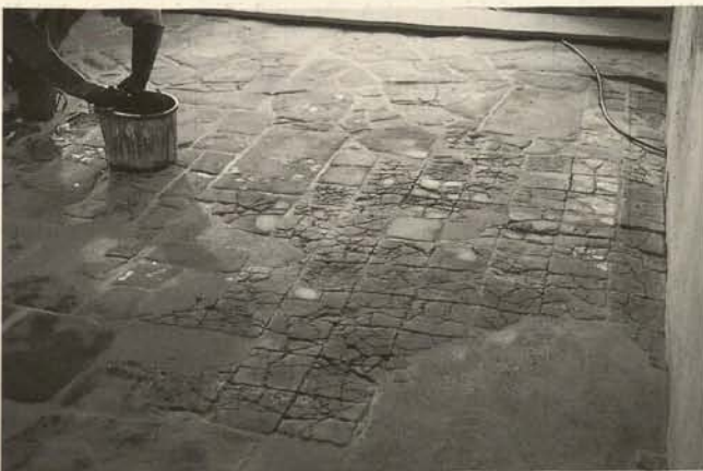
Fig. 11. Fourth case study: Acton Court. Cross passage floor after lime repairs. Note lacunae filled with mortar, and only the larger joints.
