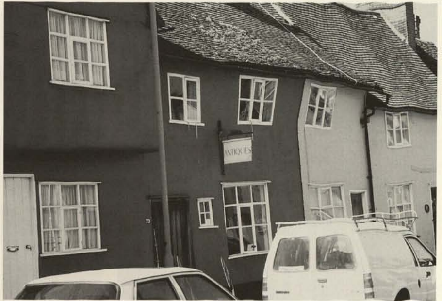
Fig. 4. Old Structural Movement ... – All old buildings move, like this timber framed one. This is part of its character. In Britain too much effort is spent on trying to correct movement that may have stopped hundreds of years ago, or on remedying faults that have to be misunderstood.
