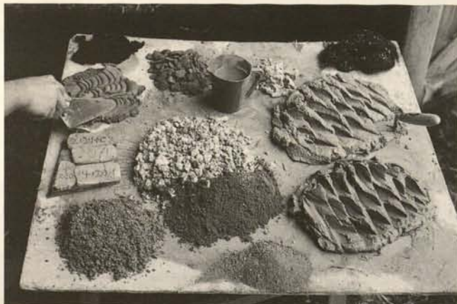
Fig. 9. Third case study: Broadfield Court. The range of lime products used on the repairs to the doorway. Note goat hair for reinforcement of mortar for hoodmould.
