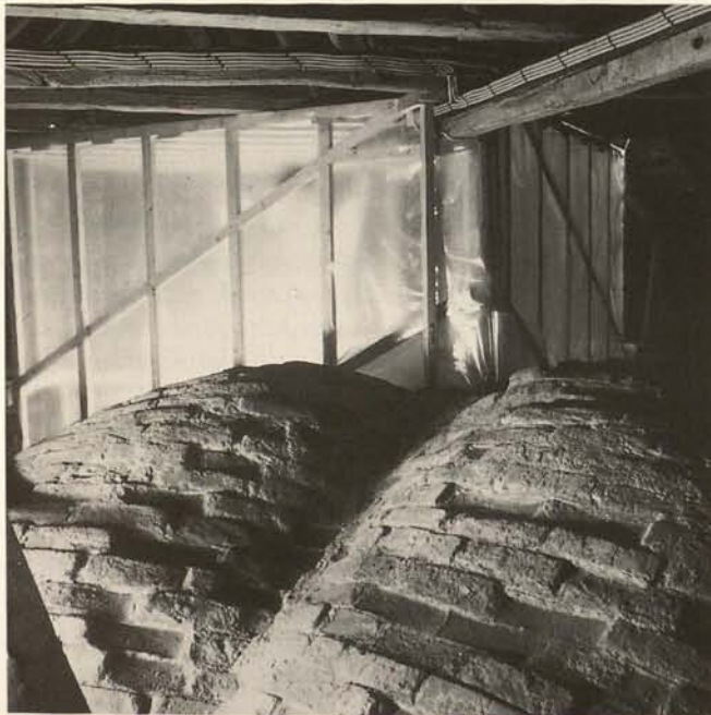
Fig. 8. Kirkerup Church (Zealand). The top side of a 14th century vault, with bricks showing deterioration caused by salts (mostly natrium chlorides).
