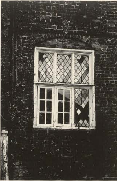
Fig. 3. Alterations to Window. – The insertion of wooden casements in part of this 16 th window, perhaps 150 years ago, adds to its interest and evoking history, and should not be removed simply on the grounds of “correctness” or “tidiness”.
