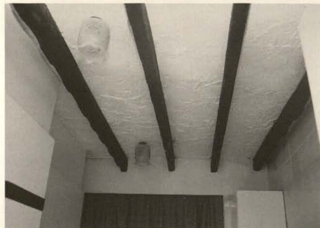
Fig. 7. Fake Beams at Highpoint. – The Society strongly opposes fakes. Here fibreglass beams have been stuck to the ceiling of one of the most important examples of a 1930s building in Britain. However they are removable.
