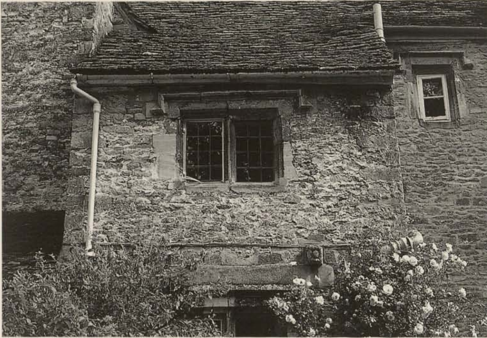
Fig. 6. Second case study: Woolgatherers staircase. The original lime surface before repair work. Note previous repairs with Portland cement on wall to right, and on timber lintel below.
