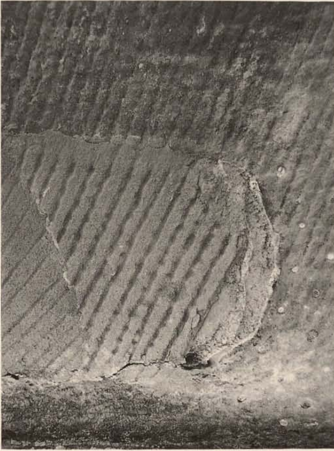
Abb. 12. Salzschiäden am Randantrag einer Reparaturstelle Fig. 12. Damages caused by salts at the application rim of a repair area
