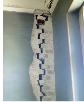
Photo 3.2.2.2 A crack on the classroom wall.
