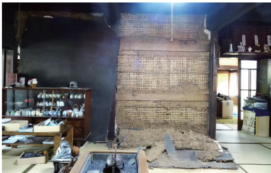
Photo 3.1.2.5 The wall of the formal room collapsed at the main building of the Yano family home ( Hontaku )
