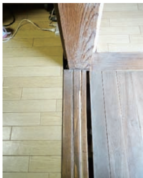
Photo 3.1.2.7 The thresholds have become misaligned at the main building of the Yano family home ( Hontaku )
