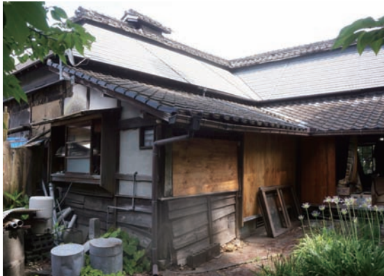
Photo 3.1.10.3 The protruding earth floor section.
