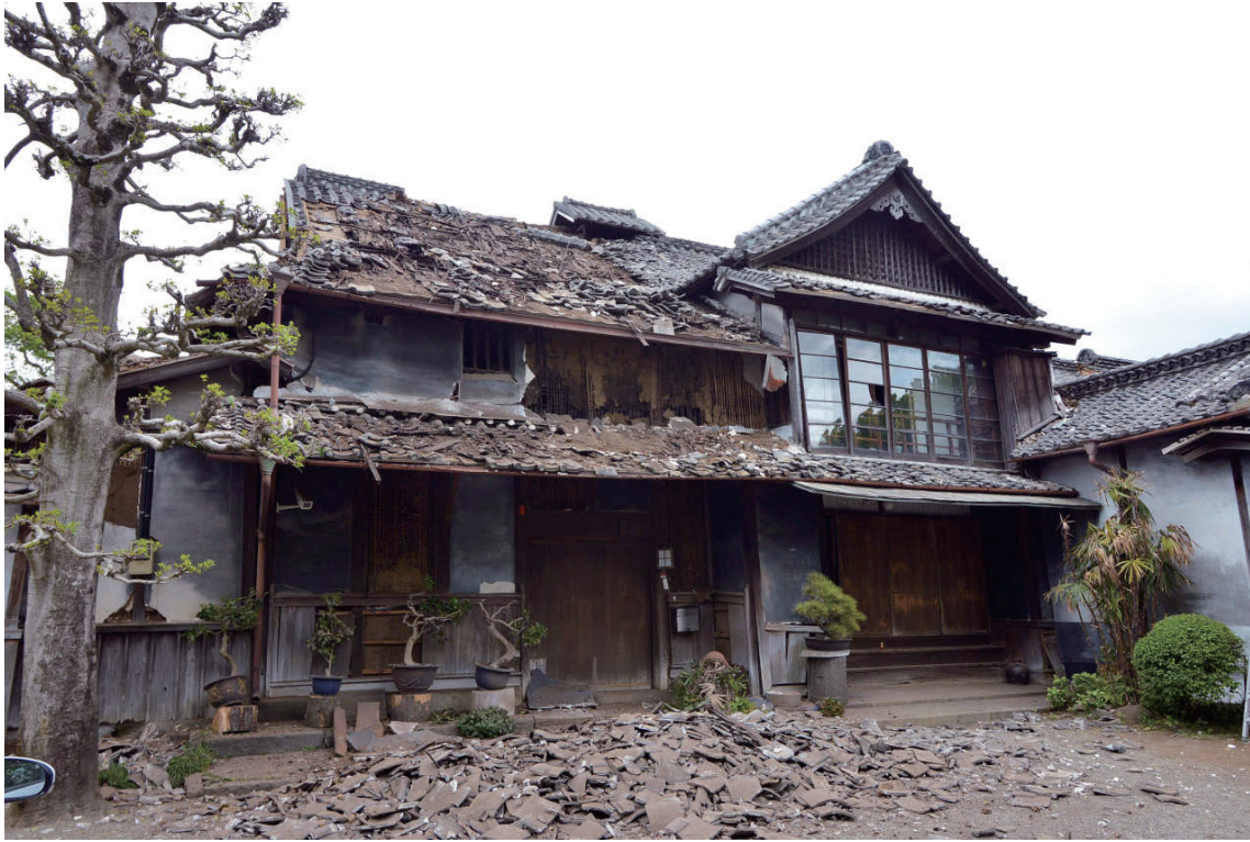
The main building of the Eto family home (Important Cultural Property), Ozu Town, Kumamoto Prefecture
