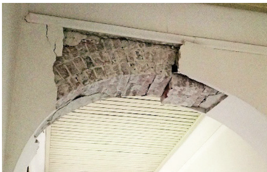
Photo 3.2.2.3 Cracks and fall down of the surface plaster on the corridor arch. (The Fifth High School Main Building)
