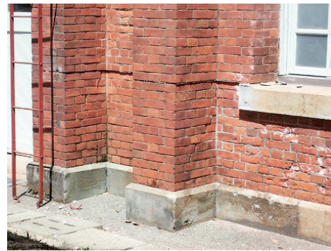
Photo 3.2.2.6 Horizontal crack at the lower level of the wall. (Kumamoto Technical High School Machine Lab.)
