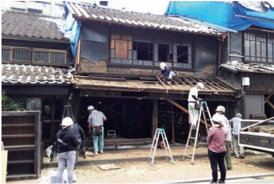
Photo 3.1.8.1 The facade immediately after the disaster.
