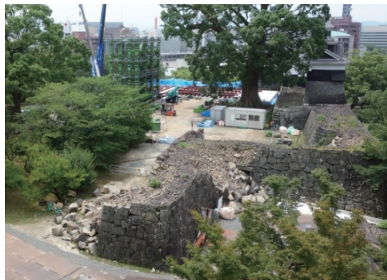
Photo 3.7.1.6 The damaged the West Turret Gate site
