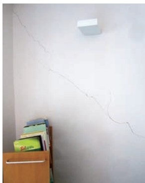
Photo 3.2.1.4 Shear cracks appeared in the walls.
