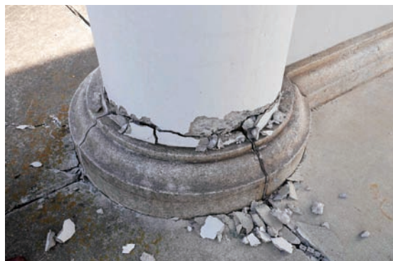
Photo 3.3.1.4 Honmyo-ji Nio-mon: damage to a column base.
