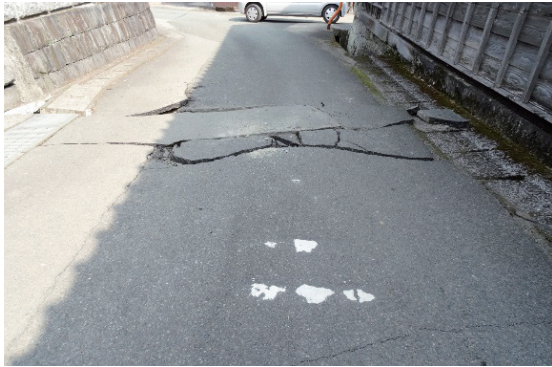
Photo 3.1.2.1 The road in front of the shed of the Yano family home ( Hontaku )
