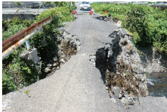
Photo 3.6.1.6 The stone wall on the upstream and downstream sides collapsed at the Zenigame Bridge
