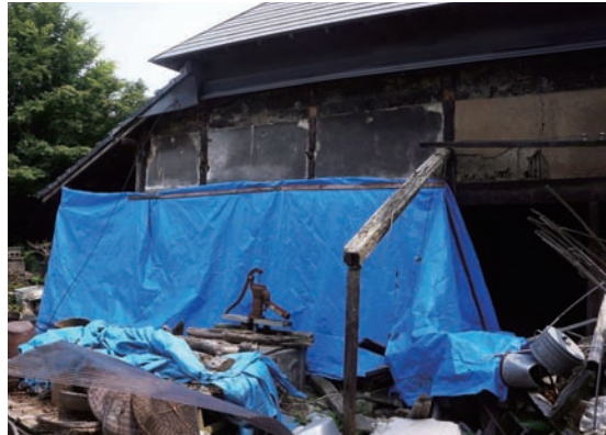
Photo 3.1.10.4 The collapsed small annex on the earth floor north side.
