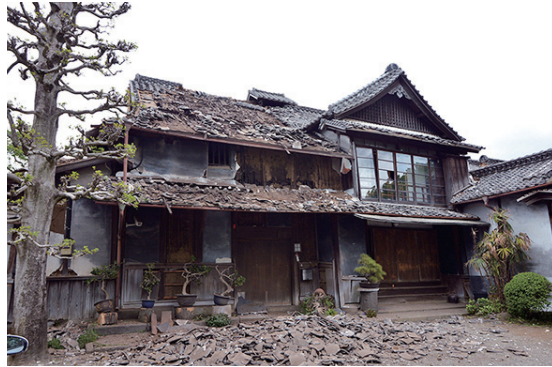
Photo 3.1.1.2 The main building (after the earthquakes)
