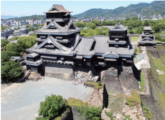
Photo 3.7.1.2 The damaged castle main keep
