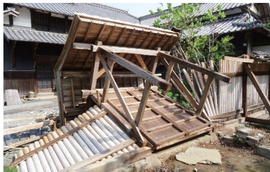
Photo 3.1.2.4 The middle gate collapsed at the Yano family home ( Hontaku )
