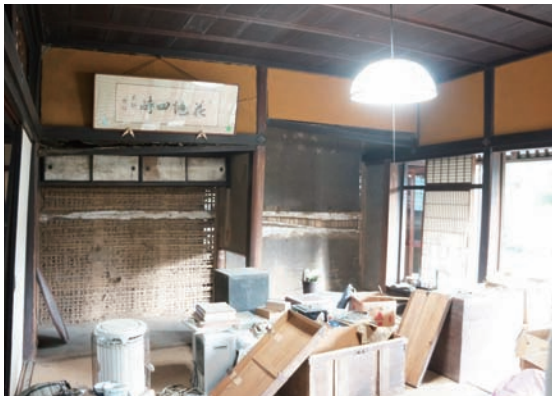
Photo 3.1.10.5 The sitting room: Collapsed interior earth wall.
