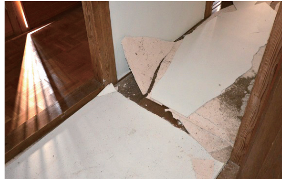
Photo 3.1.2.14 The wall's upper layer fell off at the Yano family home ( Shintaku )
