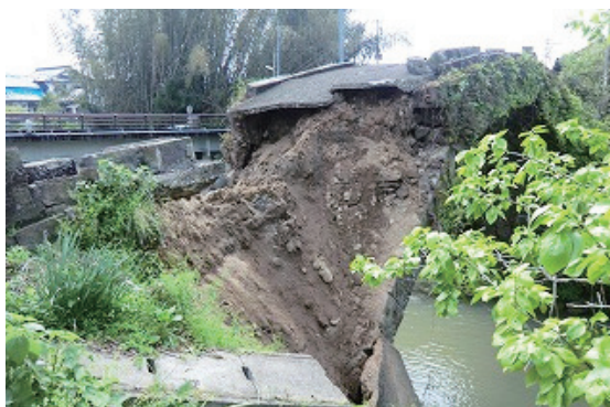
Photo 3.6.1.5 The stone wall collapsed at the Yasumi-shimoduru Bridge (Photo by Uki city)
