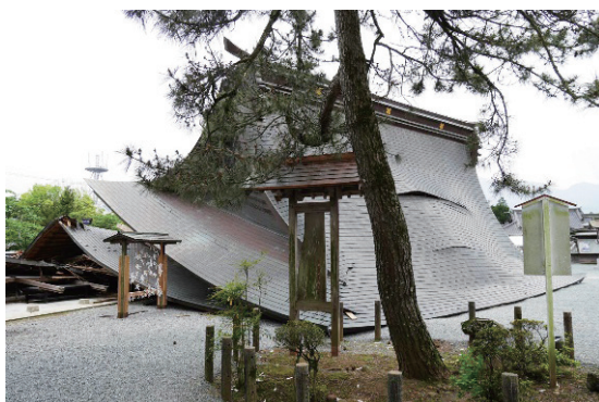
Photo 3.1.3.1 The collapsed Romon Gate of the Aso-jinja Shrine (the roadside approach).
