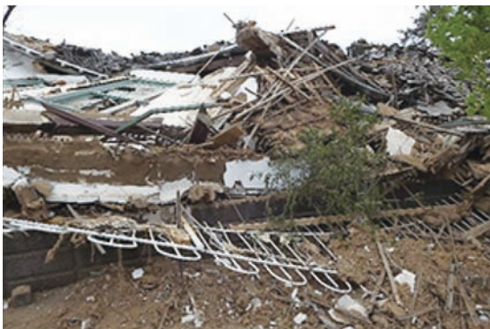
Photo 3.1.6.6 The building was completely destroyed in the main-shock earthquake (2).
