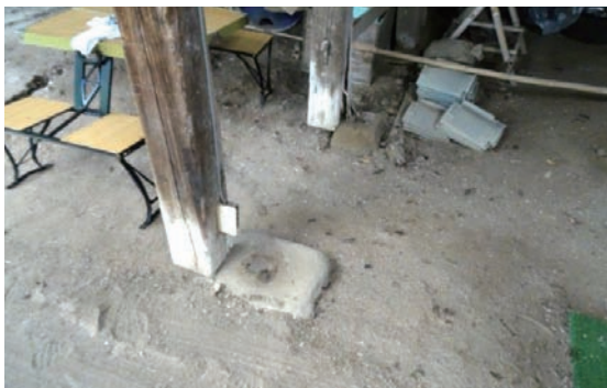
Photo 3.1.2.3 The shed pillars have come off their foundation stones at the Yano family home ( Hontaku )
