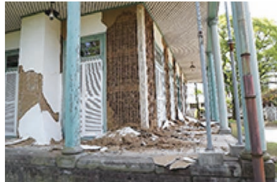
Photo 3.1.6.3 The damage caused by the fore-shock earthquake (left front).
