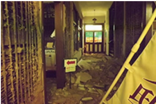
Photo 3.1.6.4 The damage caused by the fore-shock earthquake (interior).
