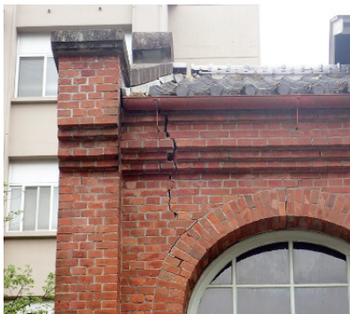
Photo 3.2.2.5 Crack on the top of corner walls.
