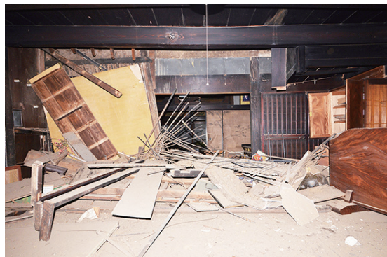
Photo 3.1.1.8 Interior of the main building, the hiroma (after the earthquakes)
