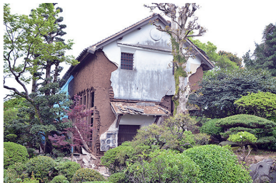
Photo 3.1.1.4 The central storehouse (after the earthquakes)
