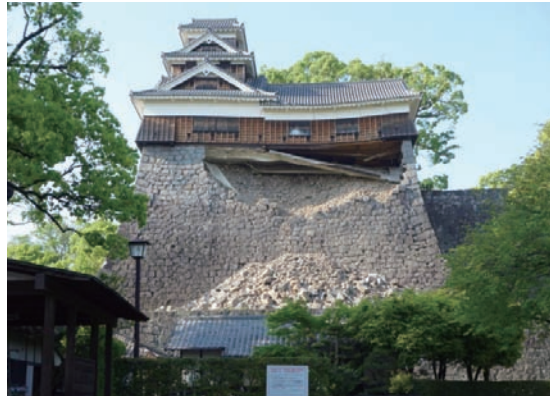
Photo 3.7.1.5 The damaged lidamaru Five-storied turret
