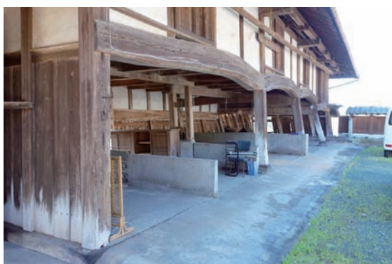
Photos 3.1.5.5-3.1.5.6 Measures to investigate the layout plan, cross section view, construction technique and structure of these vernacular architectures has carried out at the Kawabata family house before they were demolished.
