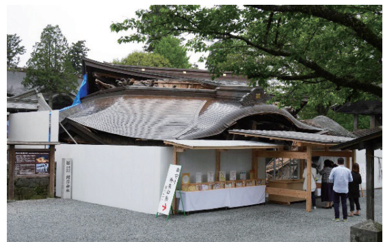
Photo 3.1.3.4 The emergency support at the San-no-shinden Shrine building in the Aso-jinja Shrine.
