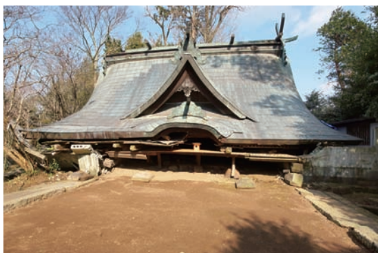
Photo 3.1.5.1 The remaining roof of worship hall of Kiyama Shrine after the earthquake.
