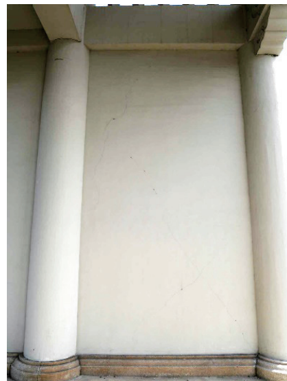
Photo 3.3.1.6 Honmyo-ji Nio-mon: shear cracks in the walls.
