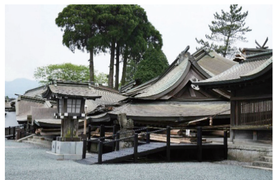
Photo 3.1.3.2 The collapsed Romon Gate of the Aso-jinja Shrine (inside the site).
