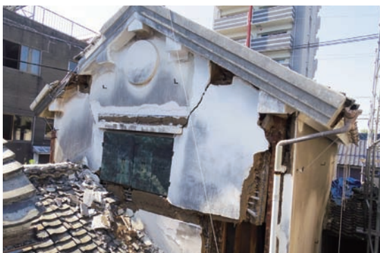
Photo 3.1.7.3 The damage to the warehouse (south side).
