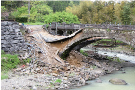
Photo 3.6.1.2 The collapsed stone wall at Futamata Fukura-watashi
