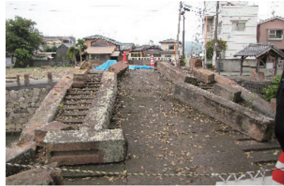
Photo 3.6.1.3 The bridge post collapsed at the Senba Bridge
