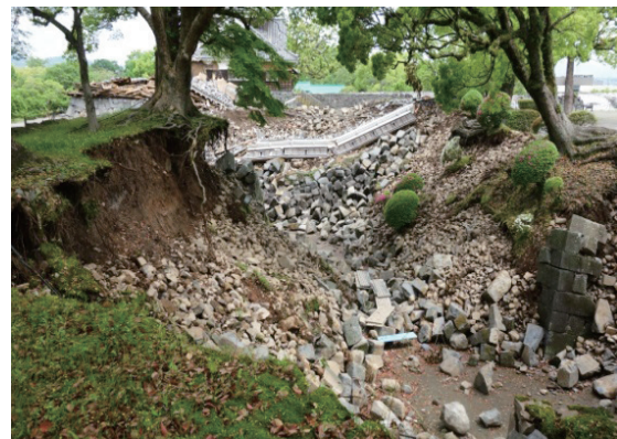
Photo 3.7.1.3 The damaged Sukiymaru Gate site (from the South)
