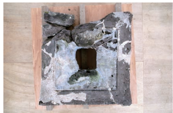
Photo 3.6.2.5 The ninth story roof with fragmented eave-ends
