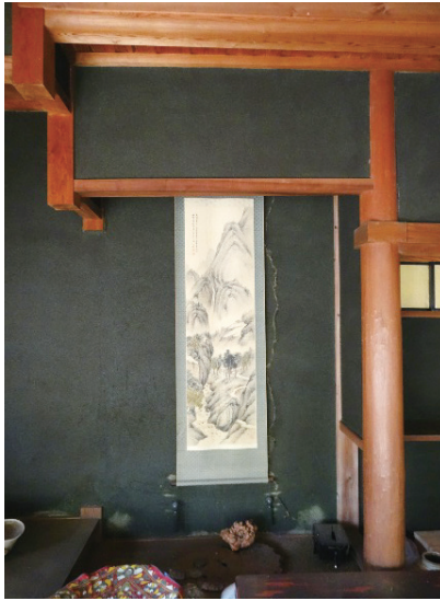
Photo 3.1.2.13 A fissure in the wall of the alcove of the Yano family home ( Shintaku )
