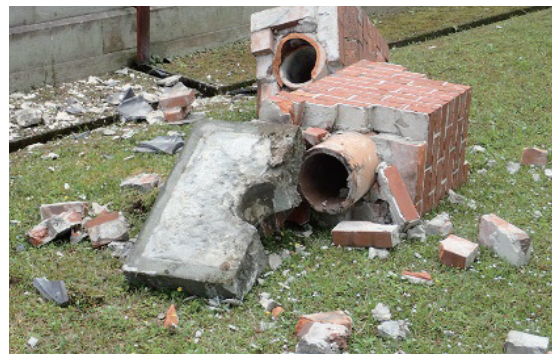
Photo 3.2.2.4 Fragments of a chimney on the ground. (The Fifth High School Chemical Lab.)
