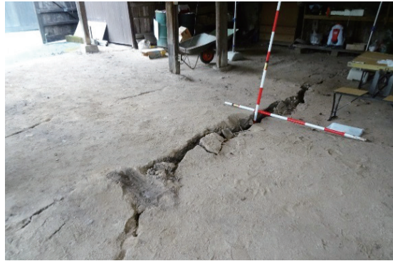
Photo 3.1.2.2 The fissure at the shed of the Yano family home ( Hontaku )
