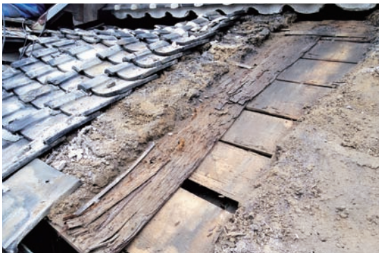
Photo 3.1.7.5 Records of the original condition before removing the roof (main building south annex).
