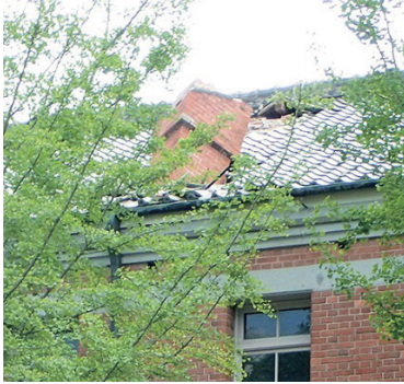
Photo 3.2.2.1 A chimney which fell down on the roof.
