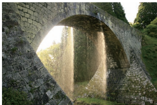
Photo 3.6.1.1 At the Tsujun Bridge, water leaked from the arch stones (Photo by Yamato town)
