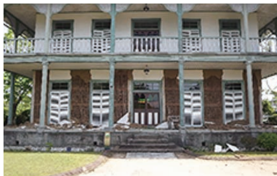
Photo 3.1.6.1 The damage caused by the fore-shock earthquake (front).
