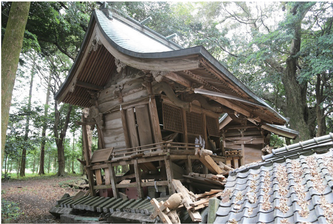
A huge sloping the main hall and collapsed the worship hall, Hachiosha Shrine
