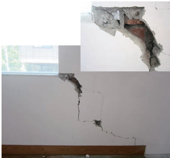
Photo 3.2.1.3 Cracks appeared around the openings.
