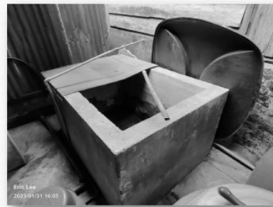
Indoor wells are used to store rainwater for drinking and cooking
