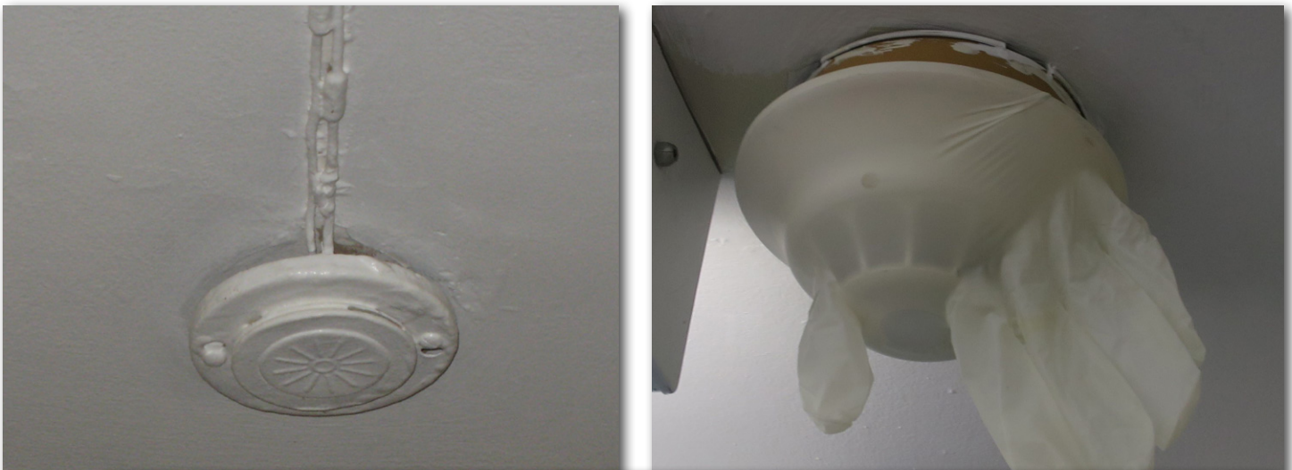
Figure 34. Fire safety systems should be frequently inspected and tested during this period, ensuring they are not damaged by construction activities (e.g., heat detectors painted, or smoke detectors covered, to limit false alarms due to dust and debris).
