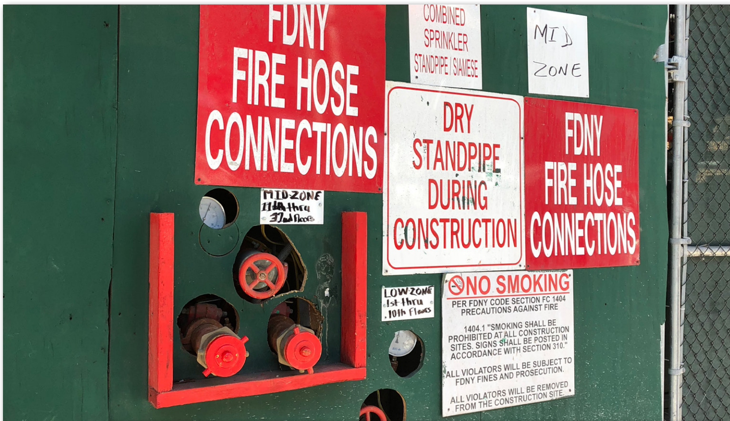
Figure 36. Temporary measures during restoration and construction should be clearly marked and simple to understand. ©Marrion Fire & Risk Consulting PE LLC-Chris Marrion
