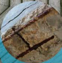
Fig 4: Exposed rebar and concrete spalling on the building's exterior
