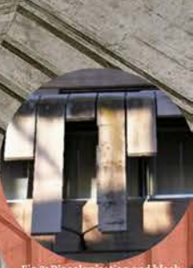
Fig 3: Biocolonisation and black crust on the building's fringes
