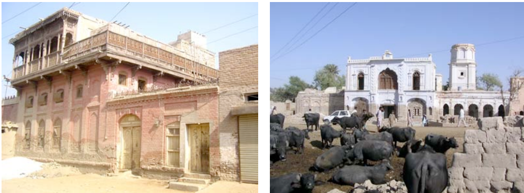
Figure 4. Havelis of Shikarpoor under threat due to neglect, abandonment, decay and demolitions.
