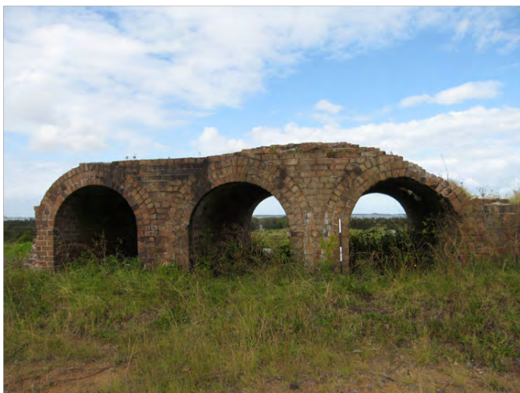
Figure 5. Brick remains of the two smelter towers featuring three arches and a platform that formed the foundations for the upper structure of the towers. This heritage element will be conserved and interpreted as part of the new development. (Godden Mackay Logan 2008)
