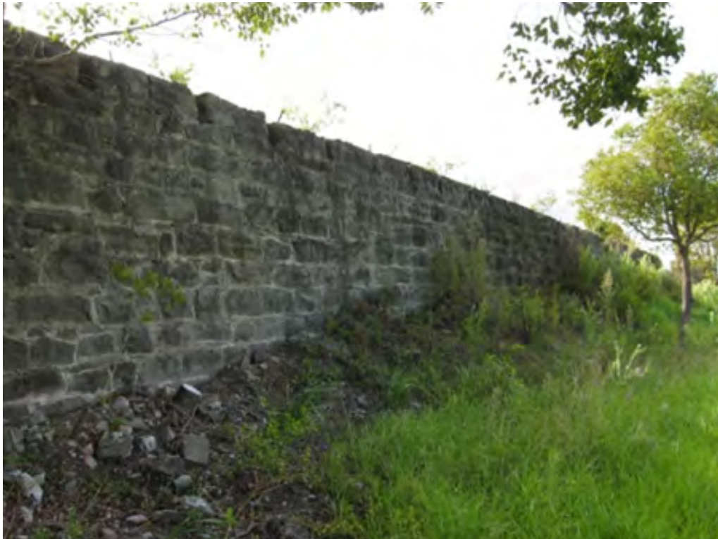
Figure 6. The eastern face of the sandstone Nickel Refinery wall will be visible from Nickel Lane, which will run parallel with the wall along its full length. This will also provide the recommended heritage curtilage. (Godden Mackay Logan 2080)
