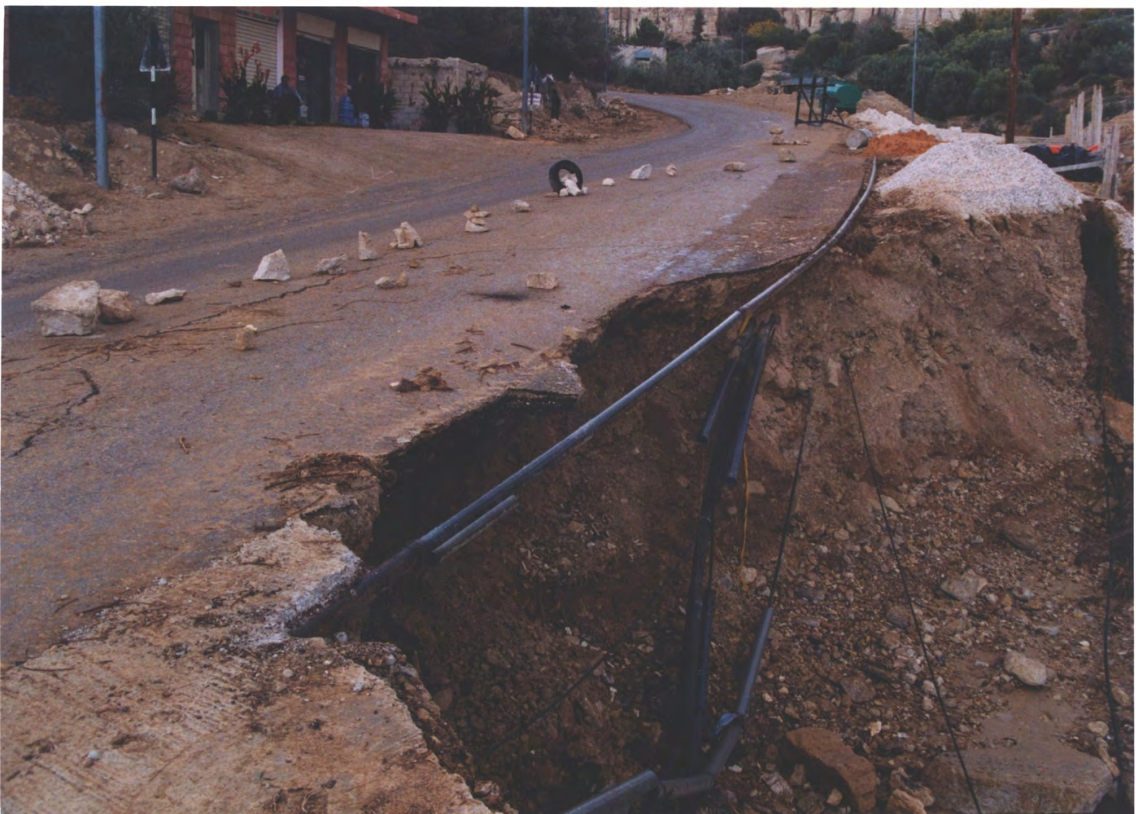
Figure 7 : Rainwater rushing over the impervious surfaces in the town of Wadi Musa produced this damage in the lower reaches of town. Two young men walking along this road were drowned, their bodies washed into the core of the World Heritage Site. Photo by Douglas Comer.
