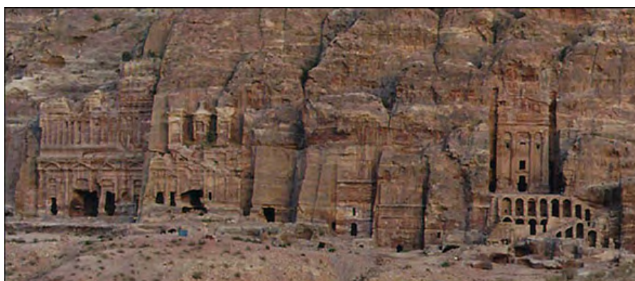
Figure 8 : Effect of salt-laden water wicking into sandstone is visible here. This kind of damage occurs from the ground up. Note keyhole shape of tomb entrances. Photo by Douglas Comer.
