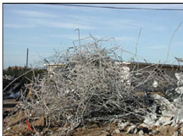
(Fig. 3) Material segregation
