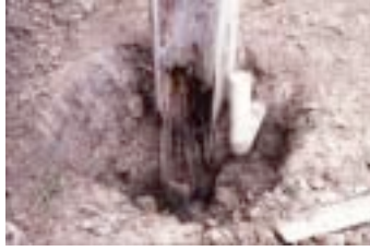
Figure 6. Timber structure damaged by wet rot & termite attack in the late 1980s.
