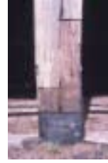
Figure 7. Spliced timber repair with a tar bandage to help waterproof the column
