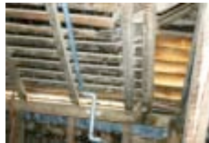
Figure 17. Carefully located sprinkler pipes.
