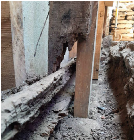
Fig. 7.a. Stone foundations and damage in bearing wooden elements in original walls (Source: Authors, 2021).
