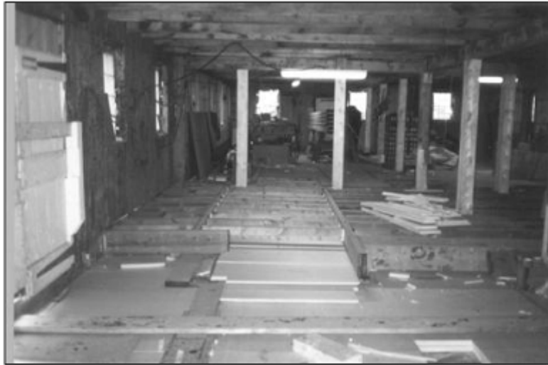
Figure 4. Conservation work on the Depot in the 1990s. Elements of the foundation were repaired and replaced, insulation was placed beneath the floor to stabilize the permafrost, and drainage was improved. (photo from Parks Canada)
