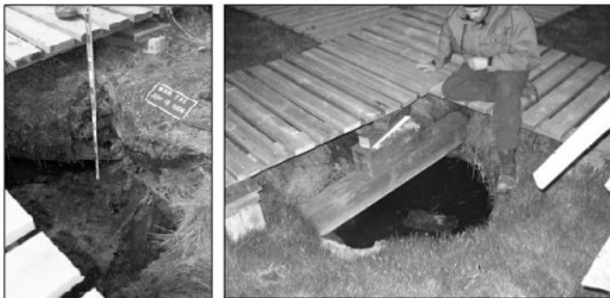
Figure 5. Sinkhole that has formed in the last couple of years within the courtyard of the Depot. The hole fills with groundwater that is warmed by exposure to surface air and then warms surrounding frozen ground. Drainage appears to be the issue. (Photos from Parks Canada and K. Skaffeld)
