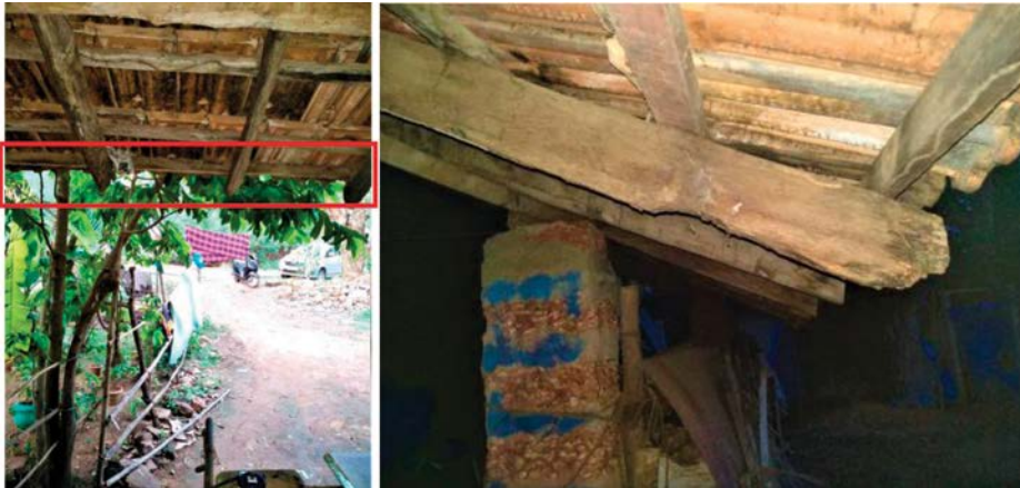
Figure 13 and Figure 14. The baton along the edge of the roof is placed with the smaller side resting on the rafters
