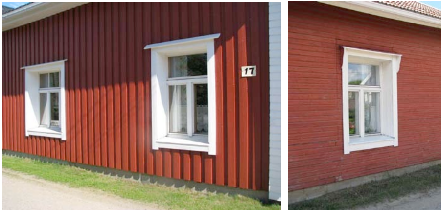
Figure 7 and 8. As an result of exterior insulation the eaves are narrower and the windows are left deep in the façade. The building has a bloated appearance. (Photos A. Soikkeli)
