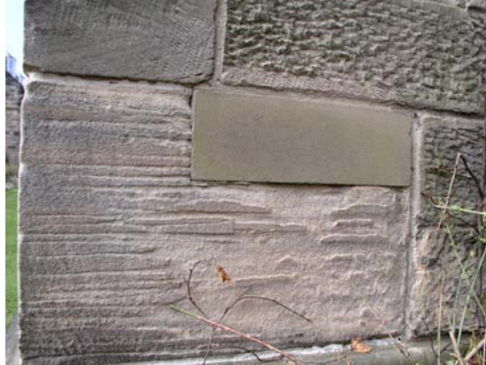
Figure 4. Accelerated decay in original masonry effected by the replacement sandstone block of different mineralogy and lower porosity.
