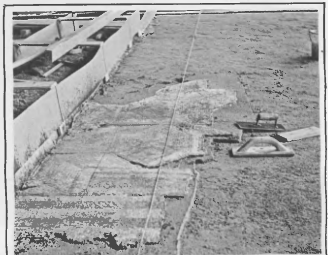
Fig. 2 - Roman palace, Fishbourne Geometric patterned mosaic being relaid. Note the grid lines being located to line across pavement from surrounding reference battens
