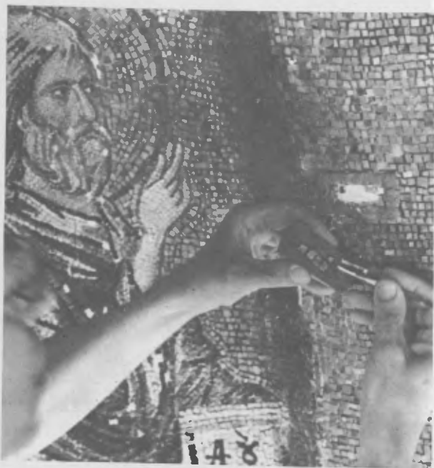
Fig. 12 - Replacing the cubes that had been removed for installation of the cramp
