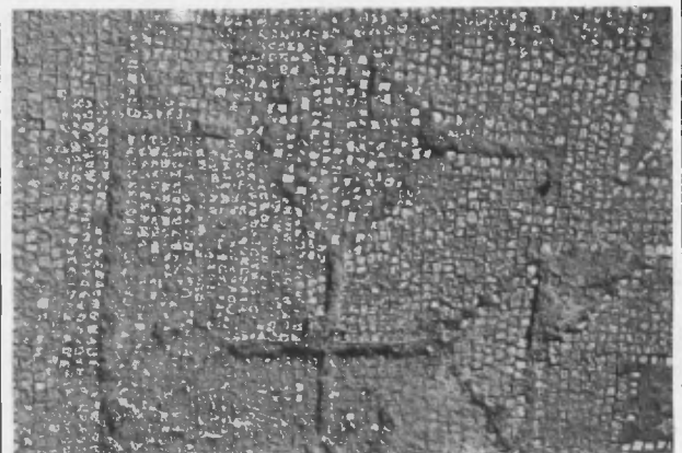
Fig. 8 - Loupian (Hérault), an unprotected mosaic in situ undergoing similar changes. Note a localized destructive process
