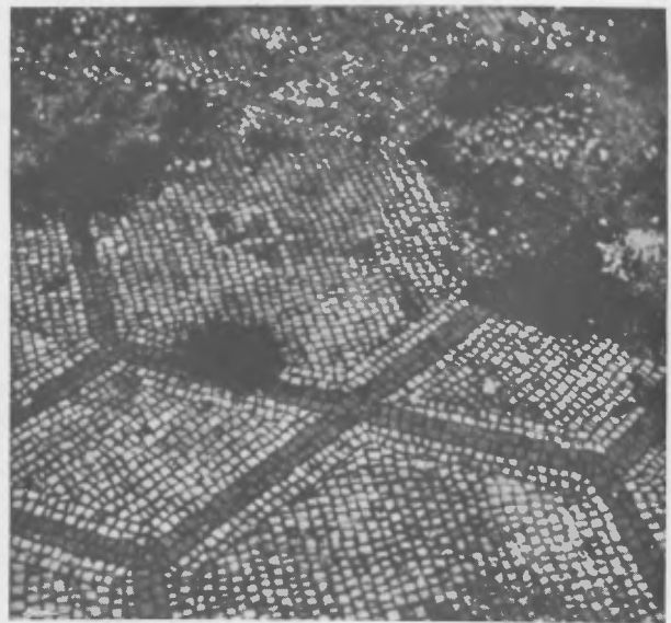
Figs. 1, 2 - Examples of damage caused by the presence of weeds
