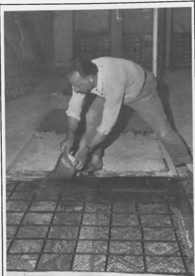
Fig. 3 - A cement mortar is applied over the metal framework attached to the back of the mosaic
