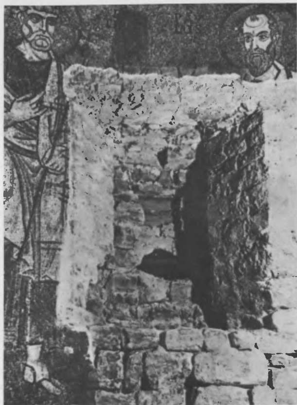
Fig. 8 - The removal of the mosaics, successive layers of mortar, and the cleaning of the underlying masonry, brought to light a series of windows which existed before the present mosaic decoration of the apse
