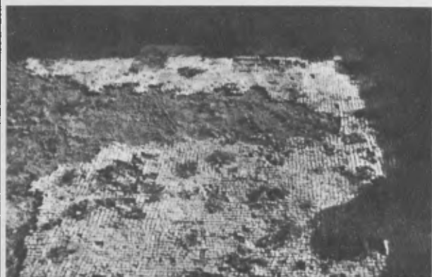
Fig. 7 - Condition of the pavement after removal of the grass. The tesserae are all clearly detached
