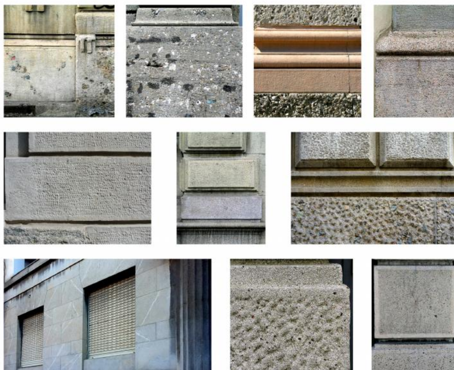
Fig. 1. Different kinds of imitation of stone (conglomerate, red or brown limestone, pink or white granite, veined marble etc.) executed using mortars made of Portland cement mixed with sands or crushed stones (early XX th Century, Milano, Italy)
