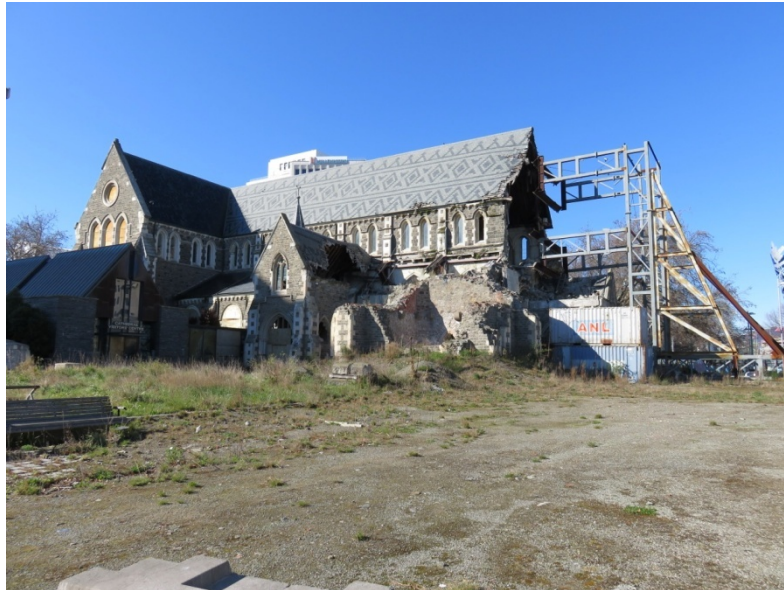
Fig.1– Christ Church Cathedral as it stood in September 2016, showing the collapse of its tower, spire, porch and western façade (Forbes, 2016).
