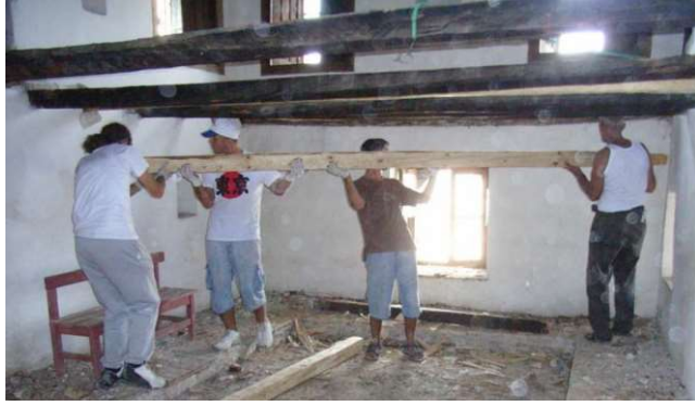
Fig.1- Participants from Kosovo, Serbia and Bosnia and Herzegovina lifting a floor joist with a Kosovan craftsman
