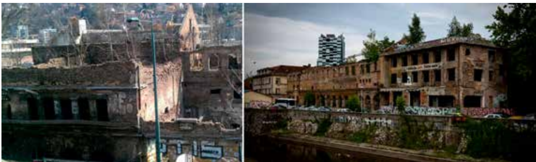
Fig. 6: a) and b) Current devastation of the electric power plant on Marijin Dvor.
