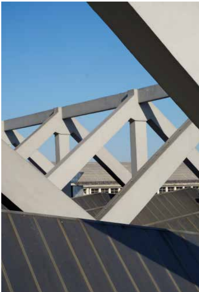
Fig 4: The suspended construction and roof structure of the metalworking plant. Photo: Miran Kambič.
