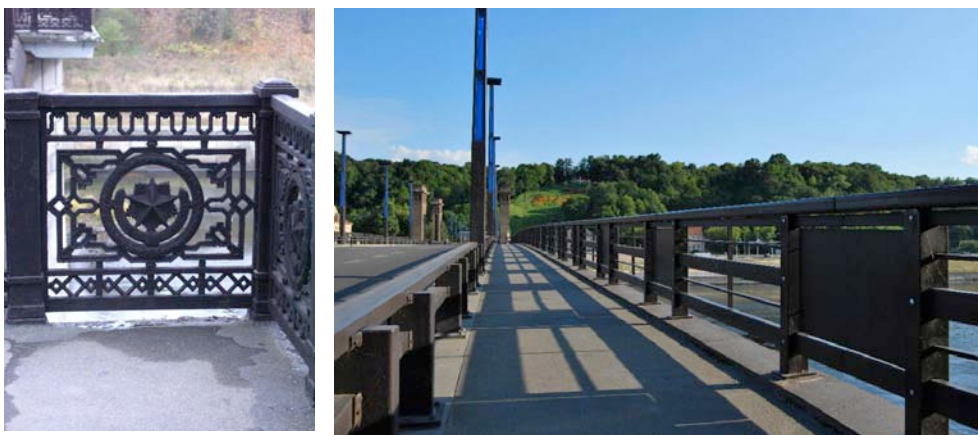
Figure 2. Bridge over the river Nemunas in Kaunas. Now and before the reconstruction.
