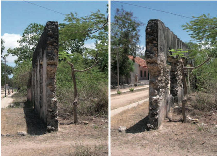
Figure 6. Wall in Rua Maria Pia. Observation of the phenomenon of disintegration where the different conservation state of the two sides (left and right) is evident and has been caused by the use of different plasters and exposure to sunlight.
