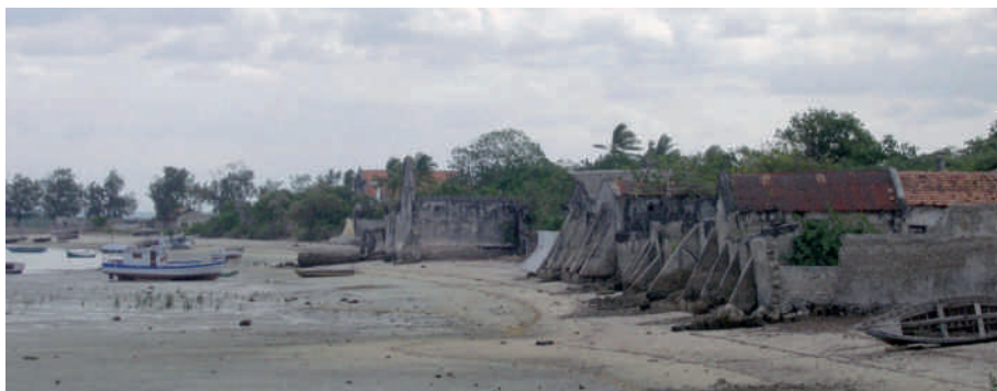
Figure 1. Porto Interior, Ibo Island. Porto Interior, Ibo Island. The buttresses prevent the collapse of the out-of-plane walls of the warehouses
