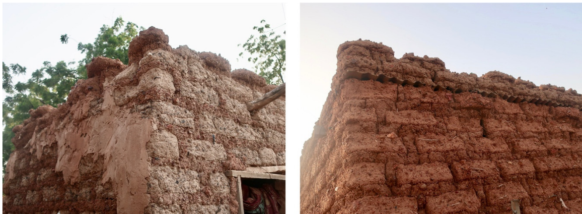
Figure 12. Material discontinuity generated by the installation of the metal sheet on the adobe wall. The change in the material used in the roof is not accompanied by a change in the construction technique, which causes the rapid deterioration of buildings.
