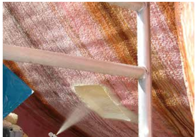
Fig. 6: Fresh foam being sprayed into the prepared voids (© adb Ewerien und Obermann)
