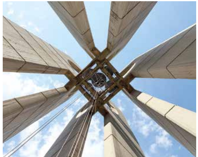
Fig. 7: The vertical body of the monument from the inside (Nikola Mihov for project ATRIUM)
