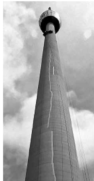
Fig. 6: Longitudinal cracks in the tower shaft
