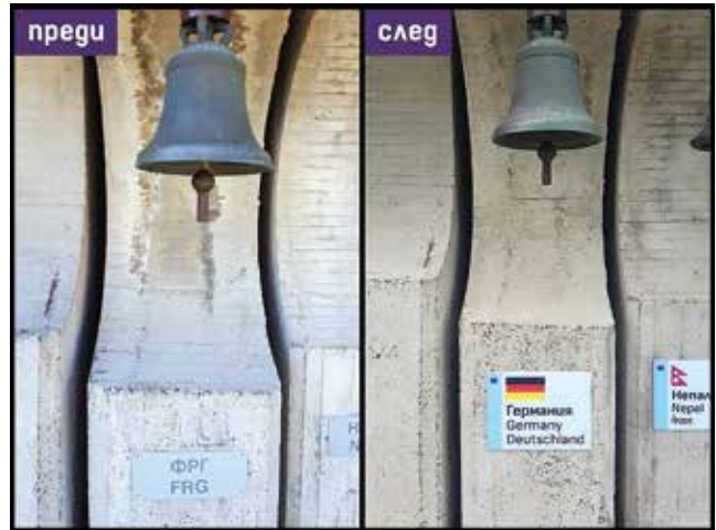
Fig. 12: Cleaning of the concrete semi-circles with bells, before and after sandblasting and labelling (Save Sofia archive)
