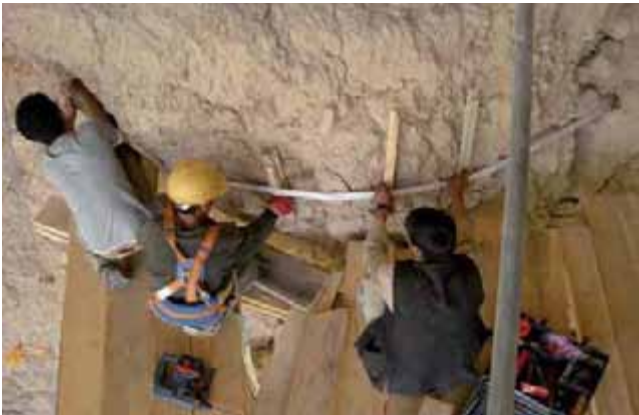
△ Fig. 3a. Provisional stabilisation of left shoulder (upper part) with tension belts
