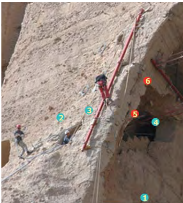
Fig. 26. The location of potentiometric crack gauges for discontinuity monitoring and alarm; in green are external sensors and red are internal to the cave
