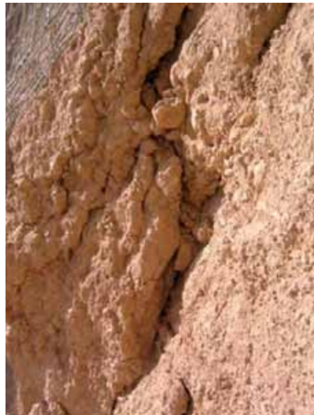
Fig. 22. Left shoulder of the Eastern Buddha (detail of an open joint containing rock debris)
