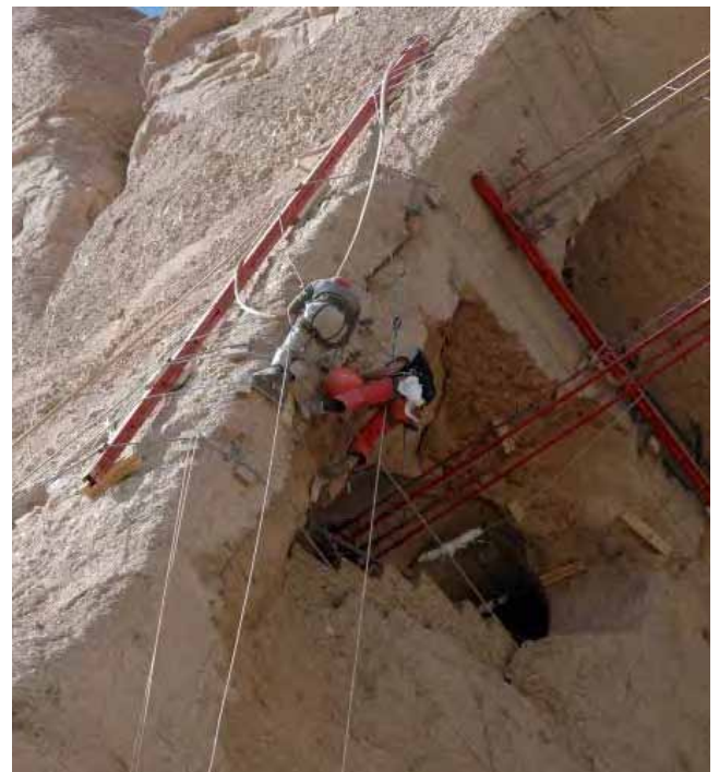
Fig. 27. The temporary support necessary for a secure execution of the work in the western wall: two long iron beams replaced in the upper part of the niche, the short iron resp. wood struts for local support and the steel ropes
