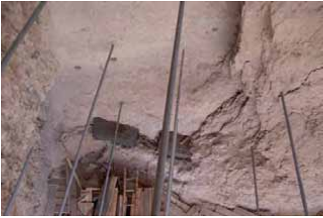
△ Fig. 1a. Right shoulder after removal of the loose rock fragments
