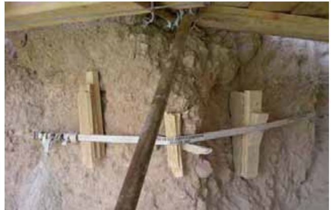
△ Fig. 3b. Provisional stabilisation of left shoulder (lower part) with tension belts
