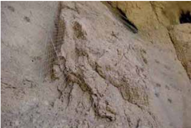
△ Fig. 2a. Head of the Eastern Buddha before removing the loose rock fragments
