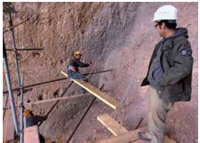
Bracket-like cantilevers are added to the scaffold so that the niche's back wall can be reached
