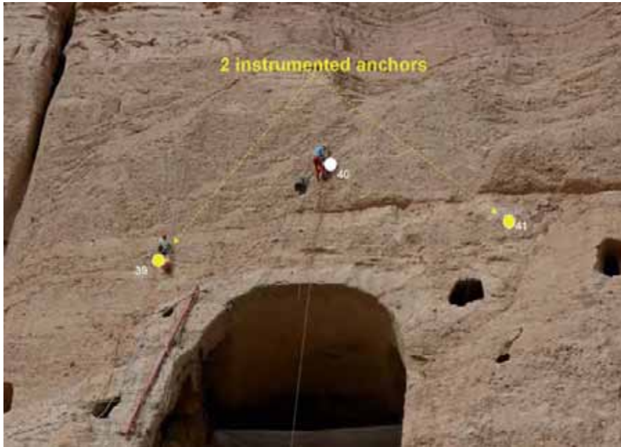
◁ Fig. 30. Position of anchors on top of the niche. The yellow ones are monitored with 10 strain gauges
