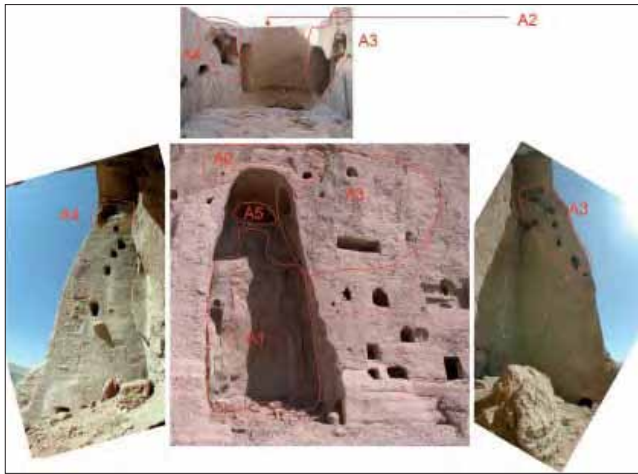
Fig. 8. Identification of the most critical instability areas in the Eastern Giant Buddha niche. The A3 block in the Eastern Giant Buddha niche exhibits the most acute instability
