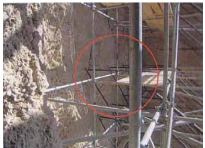
Fig. 1. Extensions made to the original scaffold consist of two grounded towers to a maximum height of about 20 meters above ground. Shown here is balcony type in the upper part. Any extensions to the scaffold reaching up higher were avoided in order to not interfere with the most unstable parts of the rock surface within and directly below the shoulder area.
