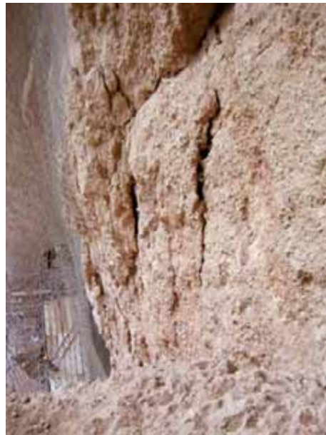
Fig. 21. Left shoulder of the Eastern Buddha (new discontinuities parallel to the back wall)
