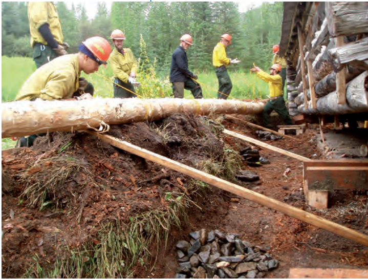
Figure 6. Alaska Fire Service firefighters installing a replacement log under Structure A, 2006. View from the east. (Photo: Collin Cogley, BLM Alaska)
