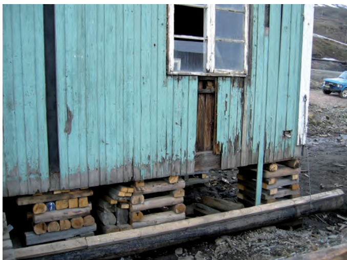
The base of a building in Svalbard had rotted from contact with soil. It has been raised up from the ground prior to substitution of rotten wood with new materials. Photo: Susan Barr
