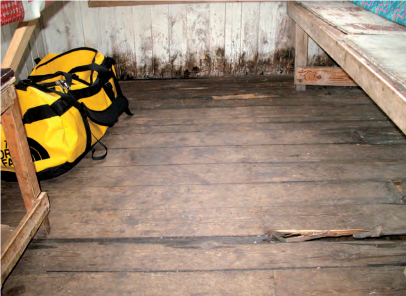
Fig. 6. A common decay area under the floor cannot be examined without dismantling.
