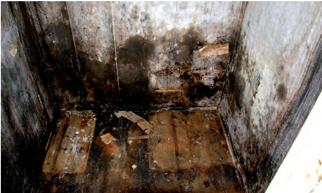
Mould and fungal growth inside a building at 80°N in Svalbard. Photo: Susan Barr
