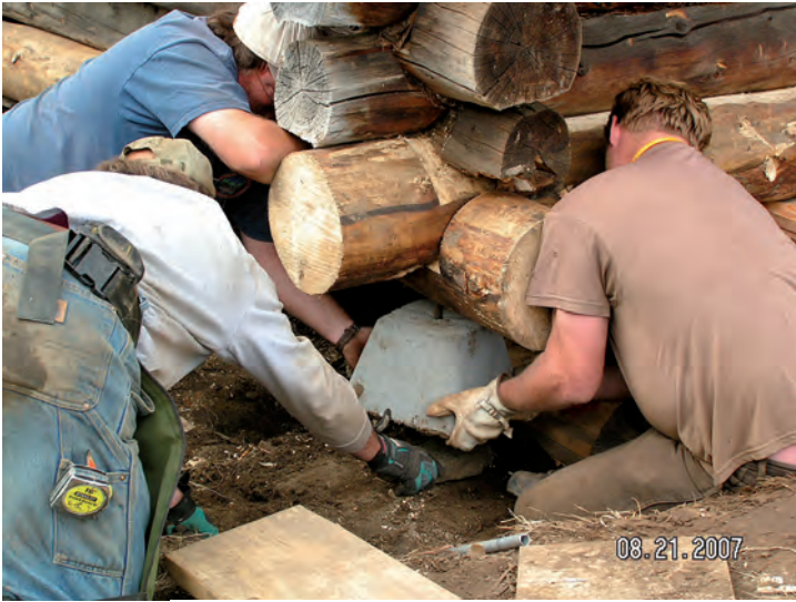
Figure 8. Collin Cogley, Eric Yeager, and Kevan Cooper positioning a concrete pier block on top of a cobble-filled pit, under the northwest corner of Structure B, 2007. The block was later hidden from casual view with soil piled up around it. (Photo: Robin Mills, BLM Alaska)
