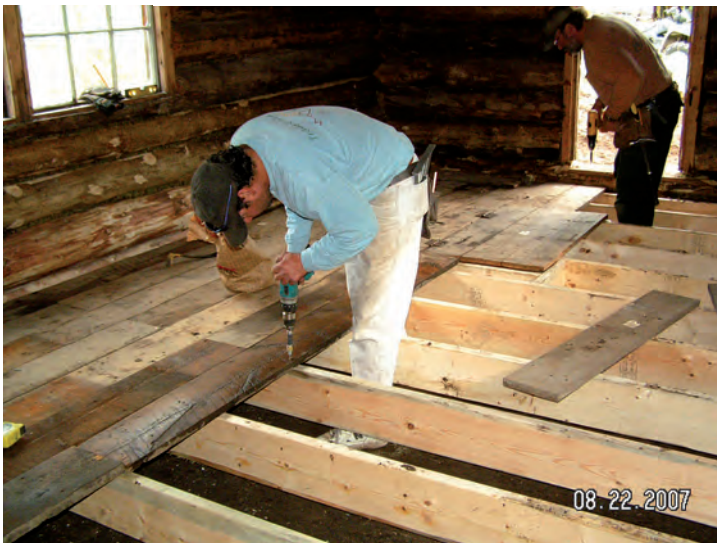
Figure 10. Tim DuPont and Eric Yeager installing a raised floor in Structure B, necessitated by the raising of the entire cabin up on concrete pier blocks, 2007 (see previous photo). Note that the original floorboards were screwed down onto the hanging joists, thus maintaining the original look of the cabin interior. (Photo: Robin Mills, BLM Alaska)
