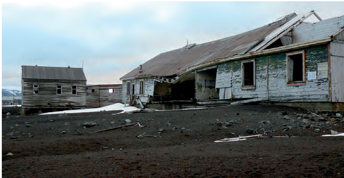
Figure 2. Structures at the whaling station at Whalers Bay are deteriorating. In addition to historic structures, there are a number of other wooden artifacts and equipment from the whaling period as well as from activities by the British Antarctic Survey located on the island that are also decaying rapidly. Photo: Benjamin Held
