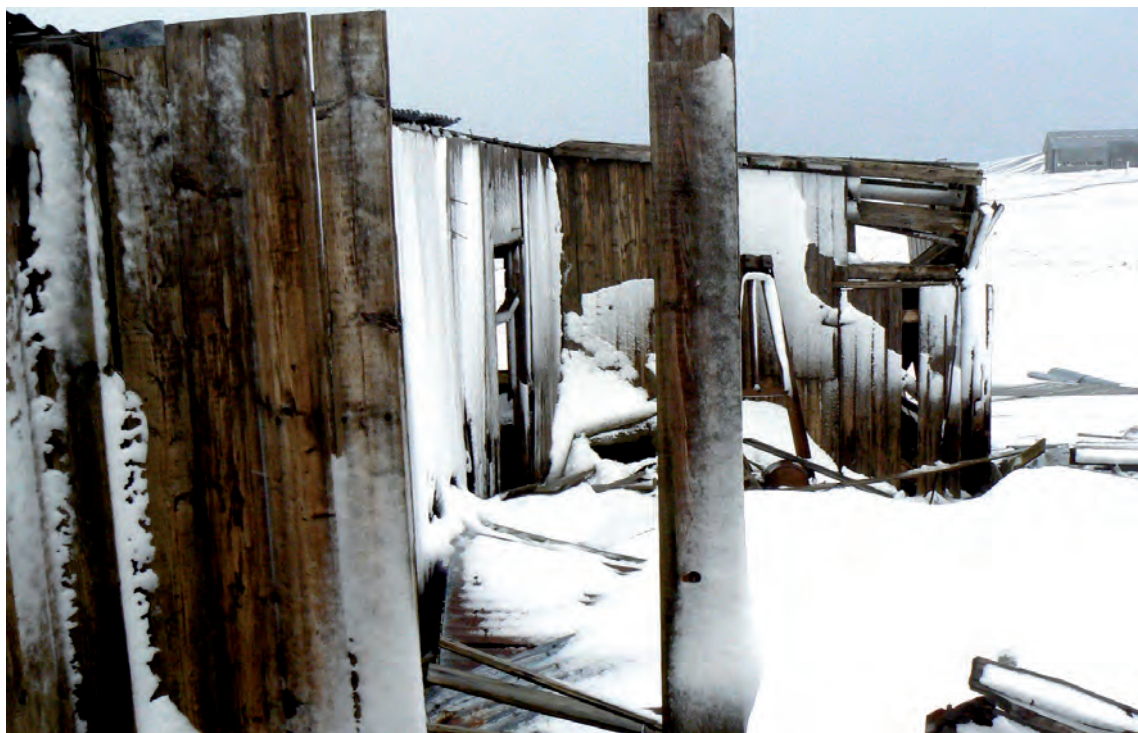
Figure 7. The north side of the dispensary at the end of a precipitation event showing accumulation of snow sticking to the wall boards. When this snow melts it is sufficient moisture to support fungal growth and decay. Photo: Benjamin Held
