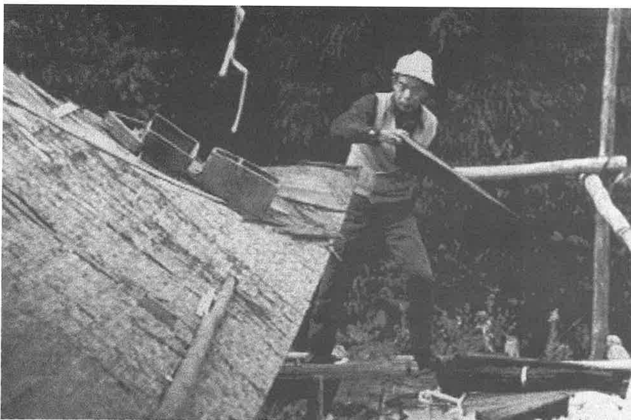
Illustration 4: Traditional roof repair in the temple of Cyojuji in Japan. Traditional skills are recognized in Japan as part of the national cultural heritage, and their continuation and survival are given special attention.
