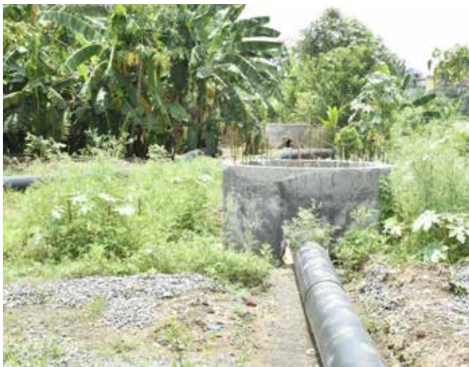
WIP for connecting sewage line to Sewage Treatment Plant near River Musa
