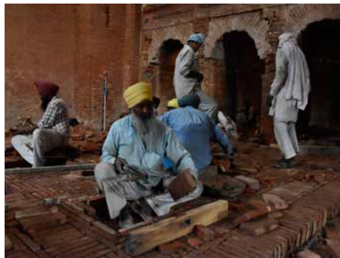
Flooring in brick tiles as part of conservation of the interiors of the Rambagh Gate
