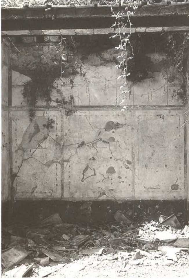
Room in a state of complete neglect, with interior wall painting already severely faded (Casa di Ifigenia).
