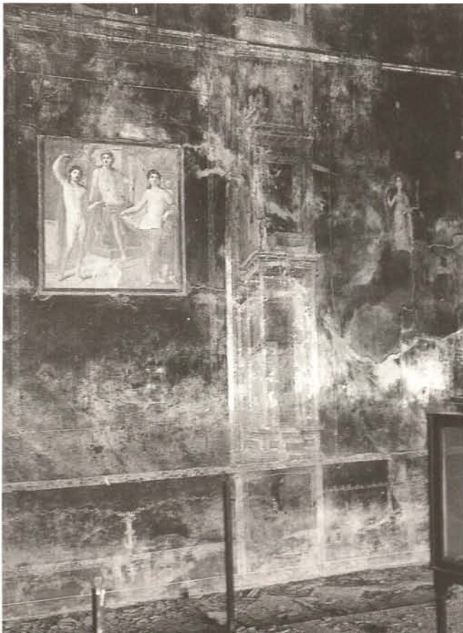
Severely endangered remains of painted wall plaster, damage caused by weathering and unprotected wall crests, as well as by vegetation (Casa dei Postumii). ▶▶
