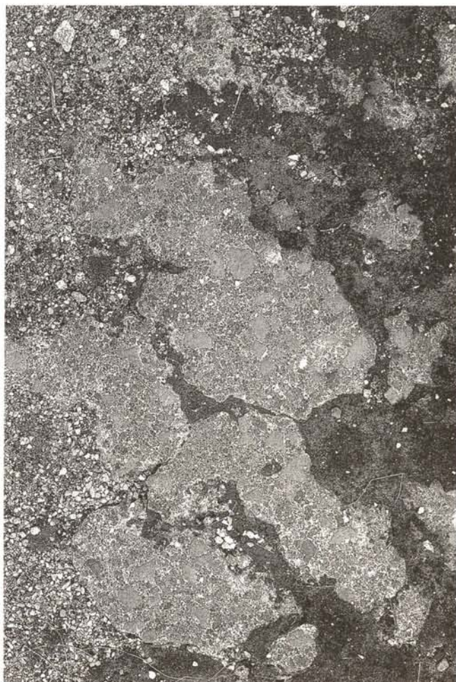
Remains of heavily damaged floors with inlaid brick fragments - the original floors in Pompeii are not only damaged by weathering but are often trodden on by the tourists (Casa dei Postumii).
