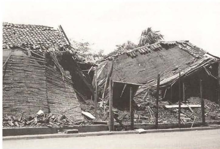
Collapsed adobe house in the historic centre of Masaya, damages caused by the earthquake of July 7, 2000
