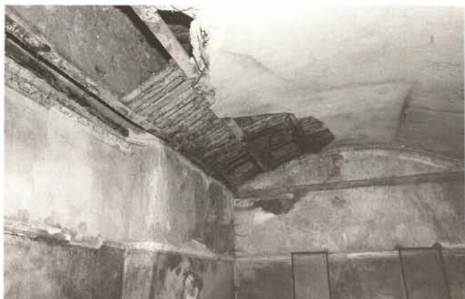
A lack of care taken during conservation measures leads to the decay of formerly well-preserved wall paintings. The barrel-shaped vault with its precious wall paintings, almost completely preserved 90 years ago, has collapsed due to a gap in the protective roof. Rapid deterioration is the consequence.
