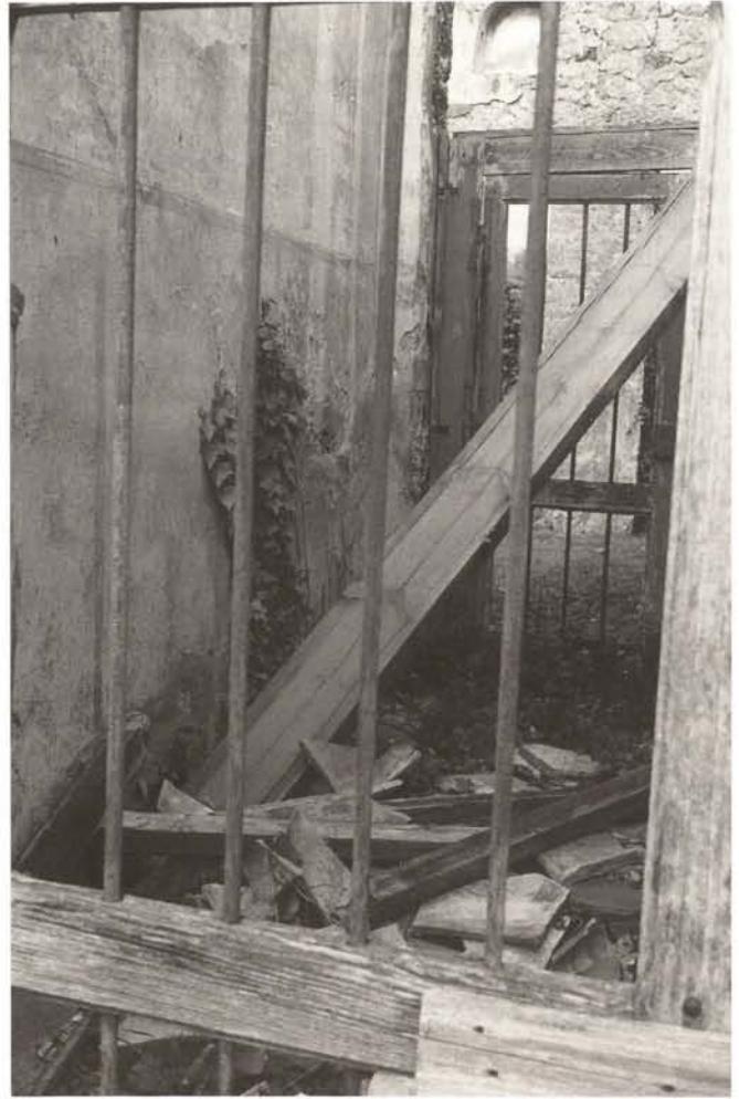
Condition of a decayed "taberna". The collapsed construction material is lying around and dilapidated. The "taberna" was excavated 90 years ago and was once decorated with well-preserved wall paintings.
