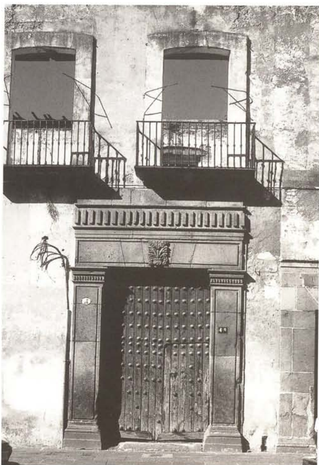
Puebla, house in the process of serious decay
