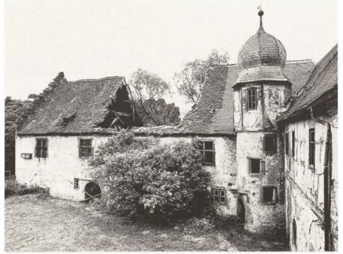
Höllrich Castle (Lower Franconia): this building, deserted for decades, is still in the process of decay despite some emergency measures.
