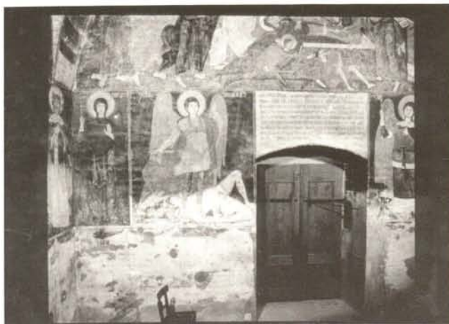
Bodjani, fresco painting damaged by humidity
