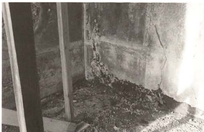
Destruction of the wall painting by moss.
