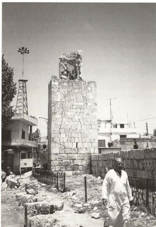
Baalbeck Great Mosque: earthquakes destroyed the upper octagonal parts of the minaret
