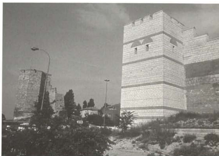
Tower 89 of the Theodosian Wall had suffered from the earthquake in 1999 (see Heritage at Risk 2000 for a photo of the damaged state). The vestiges were not enough for a proper reconstruction. A new tower has been recreated, reducing the significance and legibility of the ancient remains.
