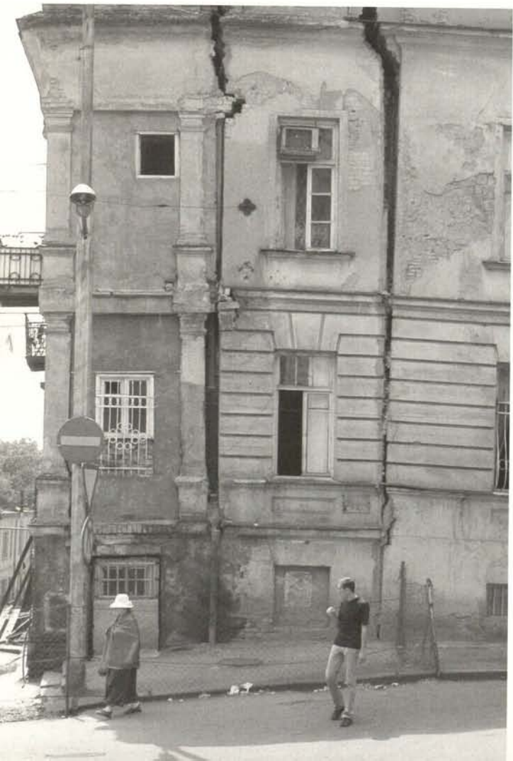
Residential house in Mtatsminad after the earthquake
