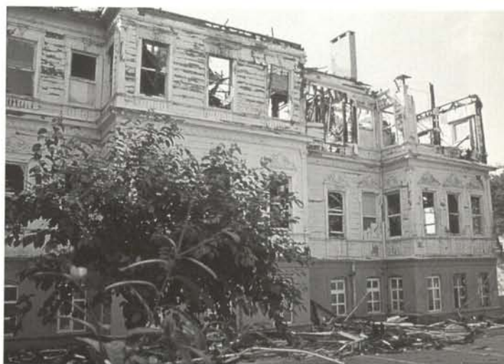
Late 19th-century timber palace on the Bosphorus, Istanbul, devastated by fire. Electrical installations in historic buildings are often the cause of such losses. Used as a public school, the building was suffering from lack of funds for its maintenance.
