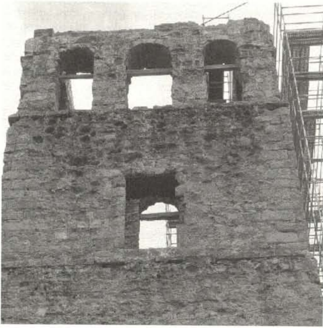
Cathedral Tower, Old Panama. National Heritage (erosion by winds and saltness, Nov. 2002).
