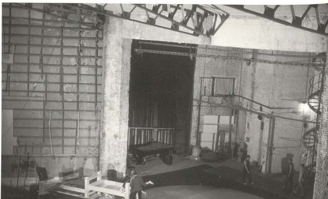
Rusakov Club. Iconic view of a still structurally strong building. The interiors are in the process of redevelopment. (Photo: N. Dushkina)
