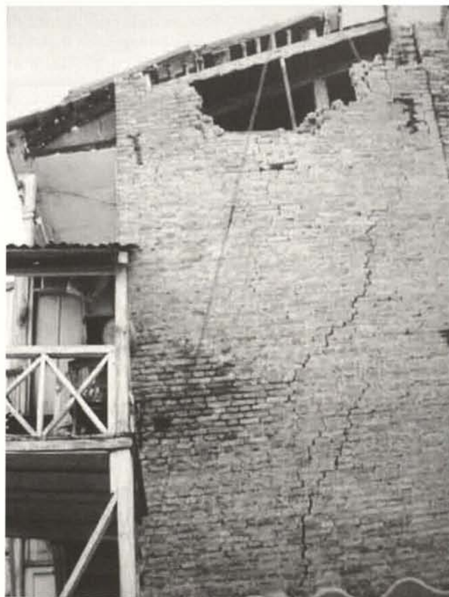
Earthquake damage in Tbilisi Historic district Residential house in Kvemo Kala micro-quarter after the earthquake
