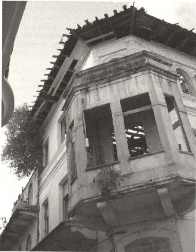
Mansion Obarrio, historic centre. World Heritage (aggressive biological attack on the structure, Nov. 2002).
