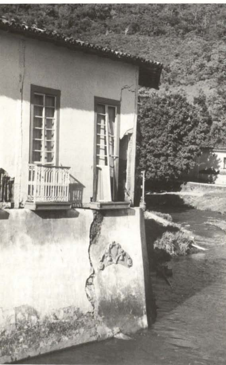
Building after flood damage
