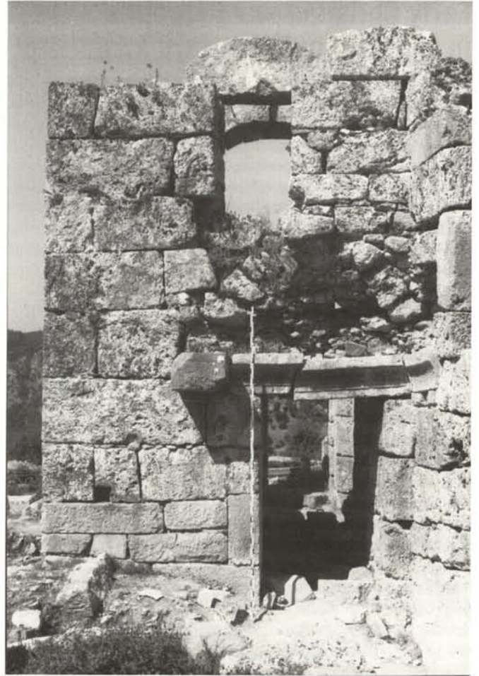
Kaunos (Hagia), domed basilica, southern aisle, eastern door – cracked lintel
