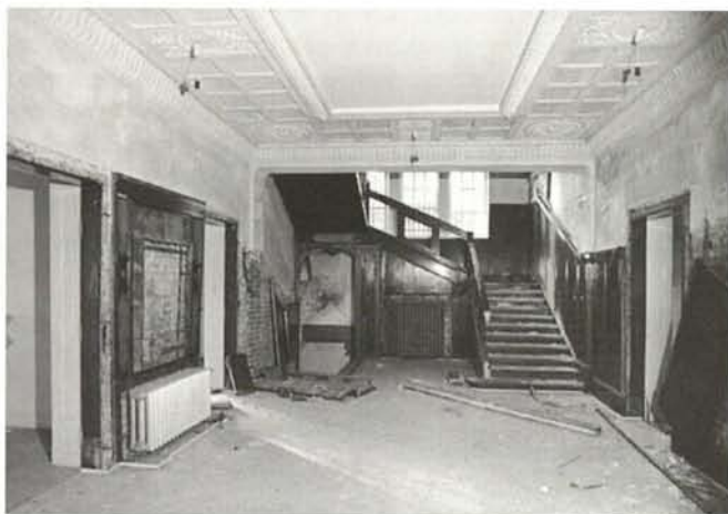
Villa in Plzeň – Lochotín Region showing devastated interior
