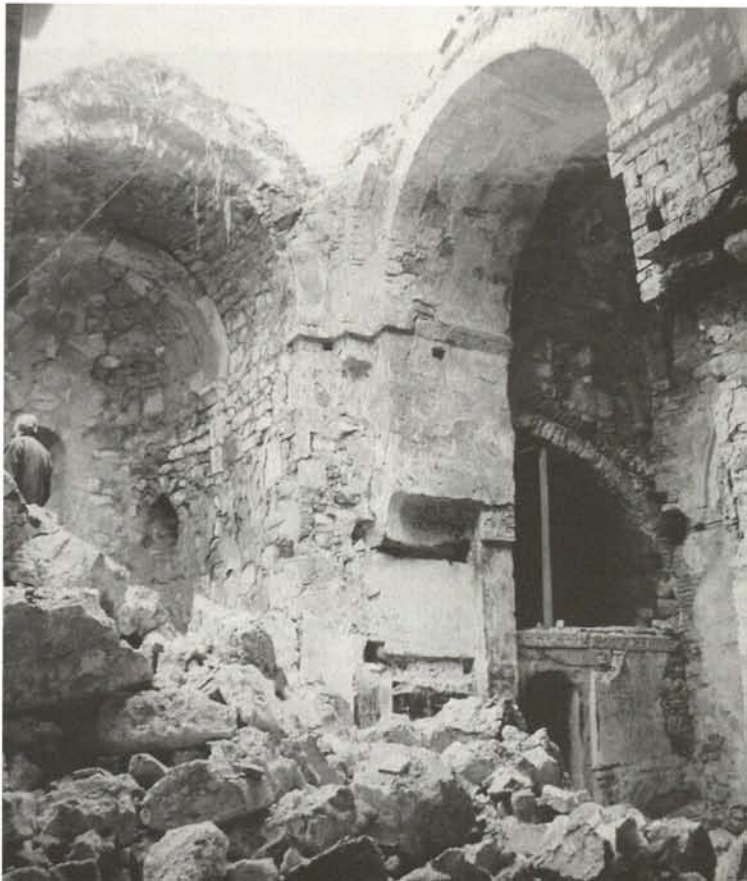
Kanchaeti Kabeni Church, general view of the church interior after the Earthquake
