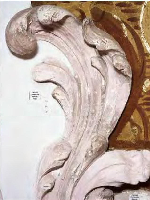
Abb. 7: Freising, Dom, Stuckdetail, Befund
