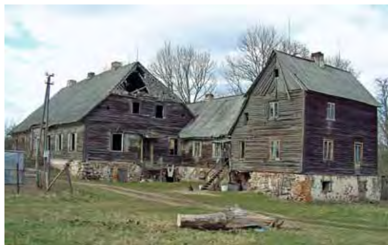
Lithuania, a timber manor house in Pavilkijys, example of a manor estate requiring urgent maintenance (about Lithuanian Manor Heritage and problems of its protection see Heritage at Risk 2006/07, pp. 108–110)
