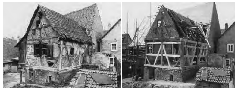
Mainbernheim (Lower Franconia), repair of a subsidiary building from 1593 in danger of imminent collapse. Due to the ruinous condition of the half-timbered walls it was decided to remove and rebuild them using stable old parts (1977/78)
