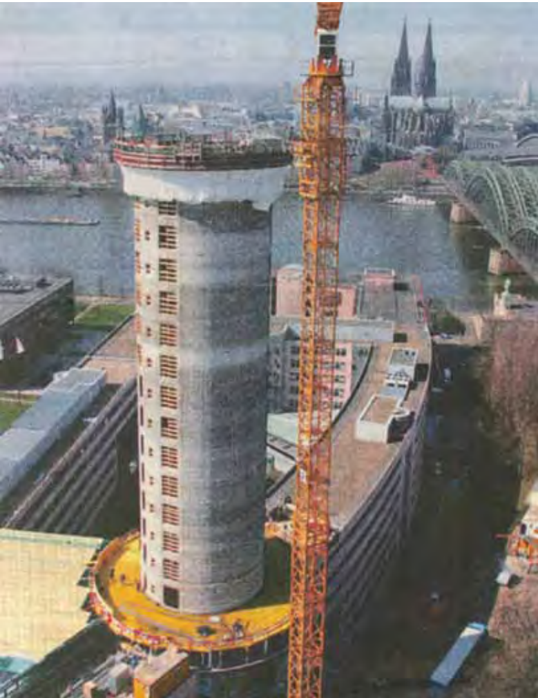
Cologne, the RZVK building during construction. The city planned a cluster of five high-rise buildings of up to 120 m which would have damaged the visual dominance of the cathedral. After the inscription of the cathedral on the List of World Heritage in Danger (2004) the project was given up and only one high-rise building already begun was erected (see H@R 2004/05, p. 73f.)
