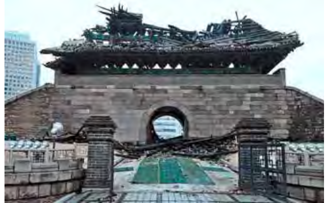
Seoul (Korean Republic), Sunghyemun Gate (South Gate) severely damaged by fire. About the exemplary restoration reusing as much as possible of the remaining materials see the report of ICOMOS Korean Republic in Heritage at Risk 2008–2010, pp. 116–117
