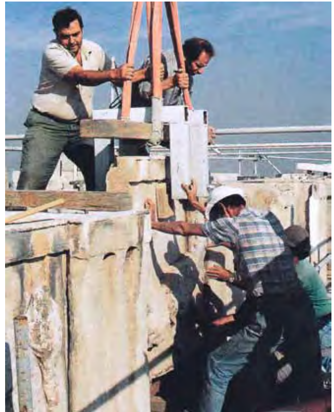
The completed corner block of the angle south-east of the cornice before its remantling
