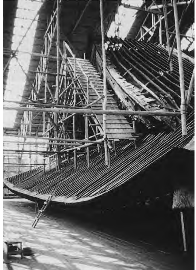
Example of traditional craftsmanship and skills in Japan: dismantling of a wooden structure in traditional scaffoldings
