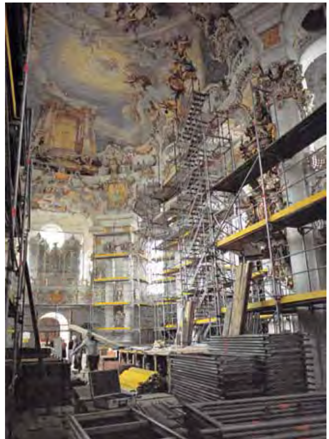
The Wies Church during erection of the scaffolding for the restoration of the interior, 1986
