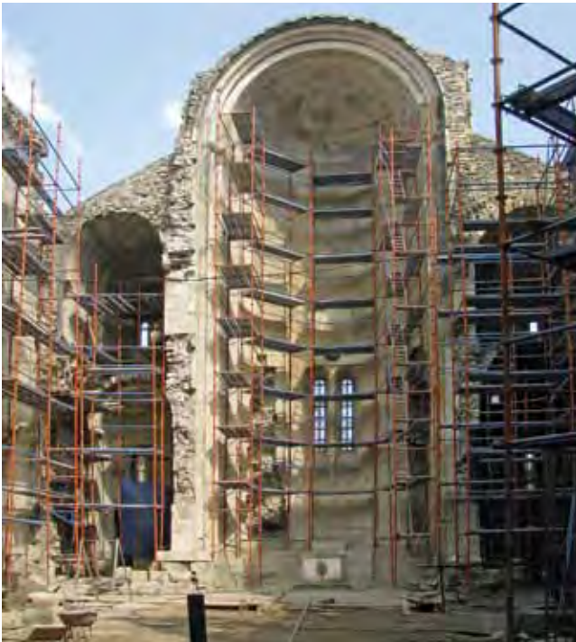
Bagrati Cathedral, Georgia. The attempt to reinforce the ruin of the cathedral, blown up in 1691 by the Turks, in the sense of an extensive reconstruction has threatened the authenticity and integrity of the architecture dating back to the late 10 th /early 11 th century (see Heritage at Risk 2008/2010, pp. 59–61)
