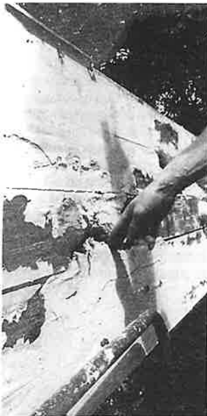
Fig. 2. The timber of the triangles was in many parts totally decomposed by fungi, thanks to the hard thick plastic paint.
