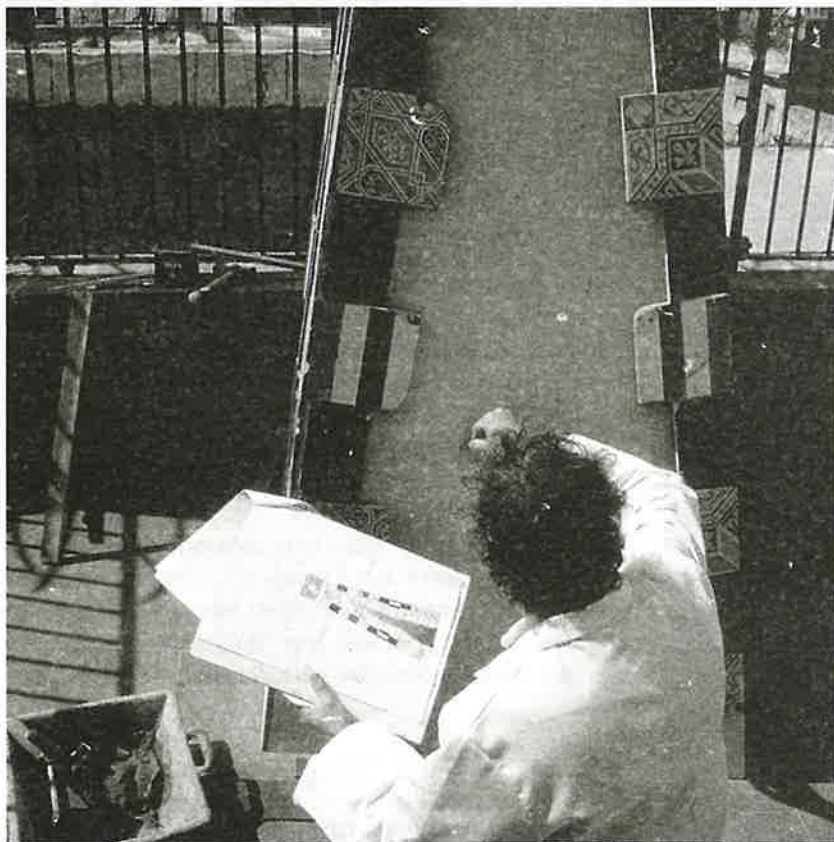
Fig. 4. The author of this article and director of the work beginning the new cladding of the shaft of the chimney Nº 6
