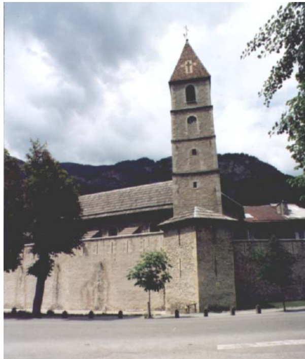
Fig. 1 External view of the Saint Martin church and damages on the vaults
