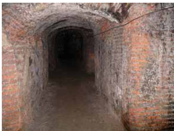
Fig 10 17th century tunnel, lined in brick and deformed by the pressure of the land.
